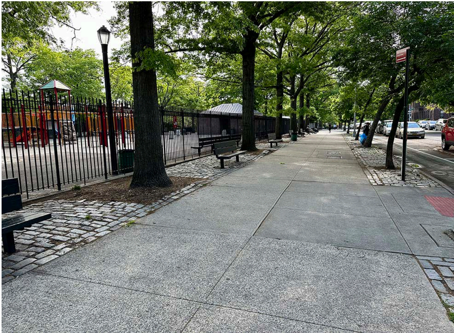
1 - Double gate and 7'-0" ht. steel fence along Skillman Ave, mature street trees surrounded by granite block, sidewalk cracked & heaving.
