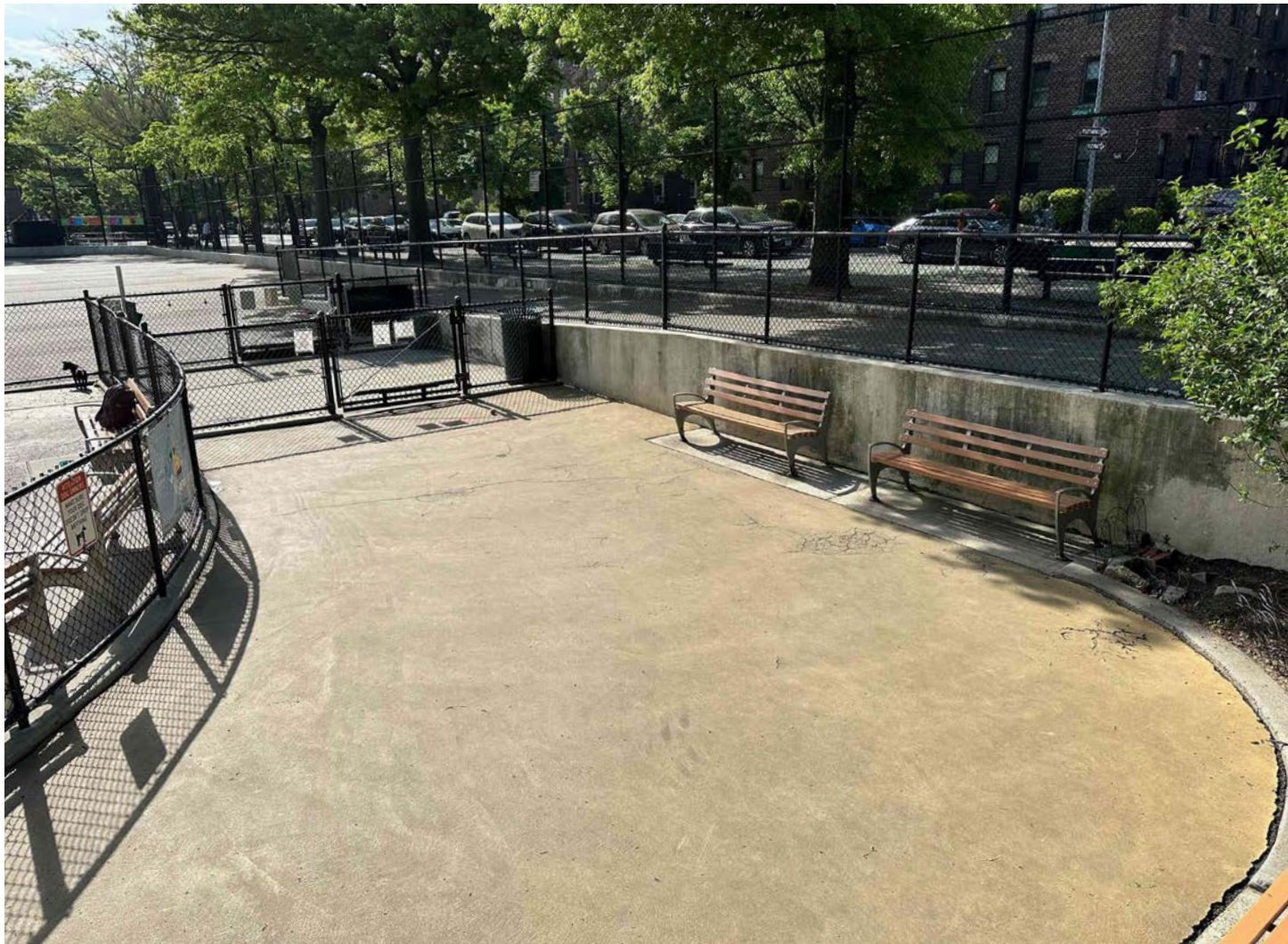
9 - Small dog run with benches, cracking asphalt pavement with color seal coat
