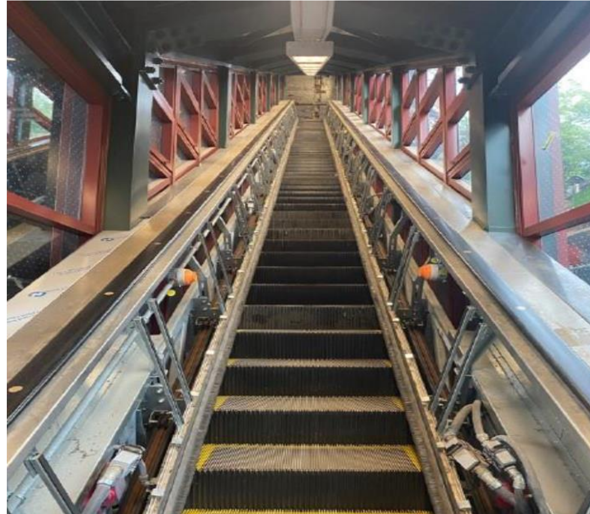
New Escalator under Testing & Commissioning
