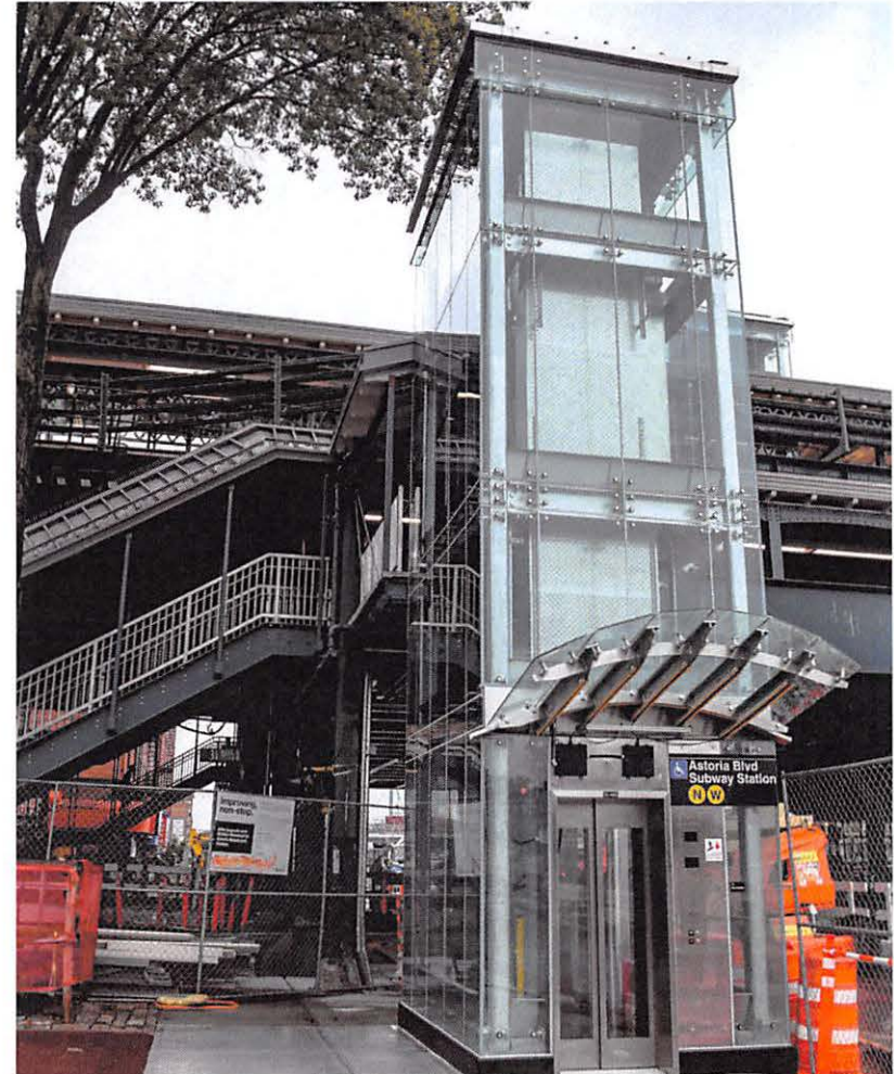
Elevators opened at the Astoria Blvd. NW Station in July 2020
