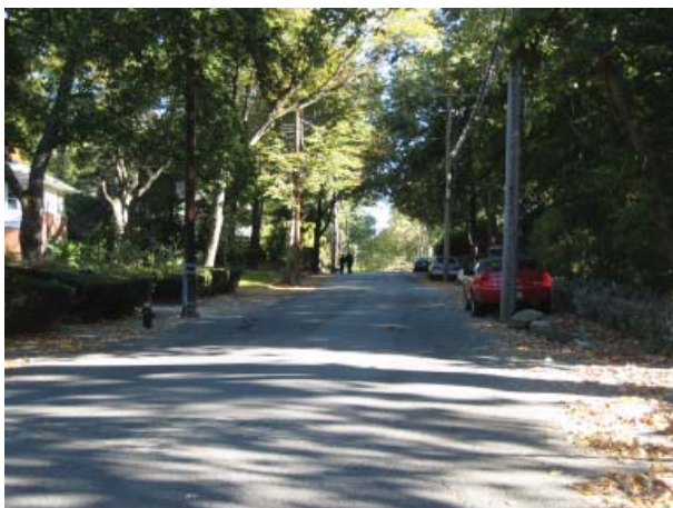
Roadway conditions along W. 254th St.
