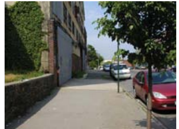
15-foot sidewalk along manufacturing uses just south of Rainey Park. Uneven pavement conditions.
