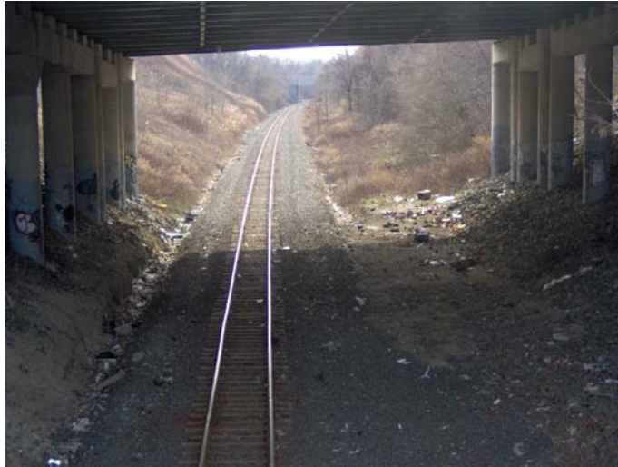
Parcel Q6305 looking south from 57 th Avenue. The Long Island Expressway crosses over above.
