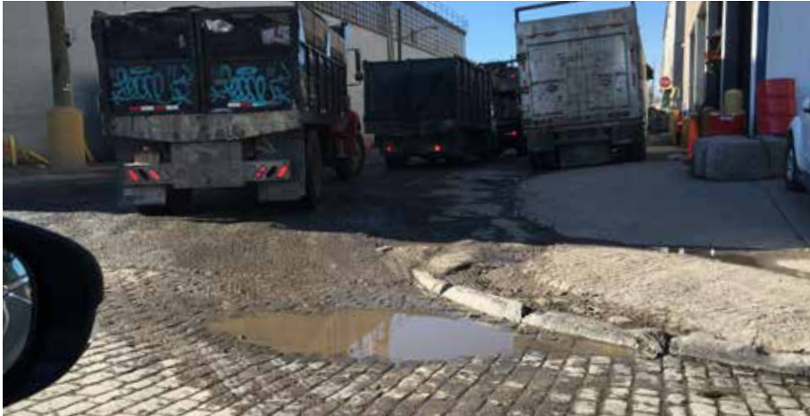
Potholes in areas with heavy truck usage
