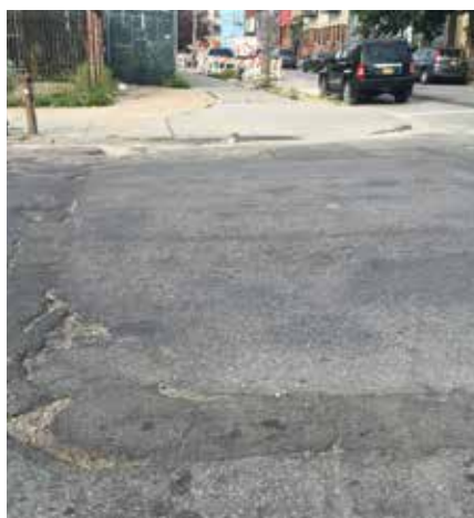
Poor roadway condition
