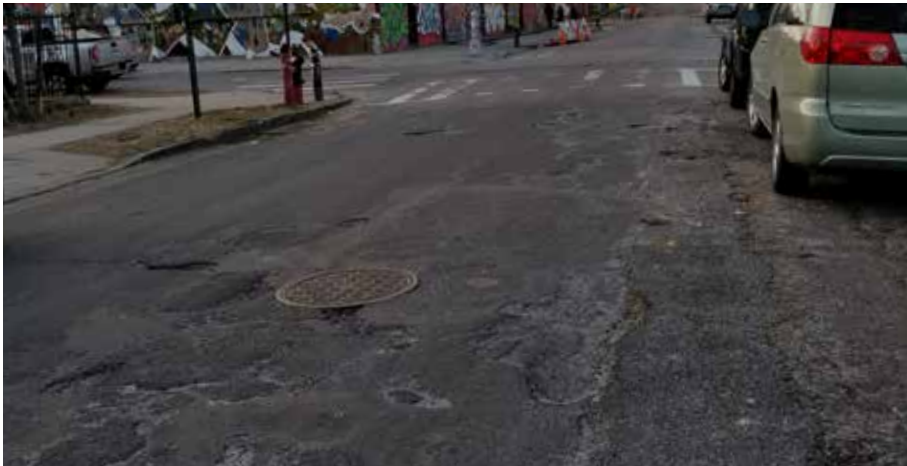
Roadways in need of resurfacing
