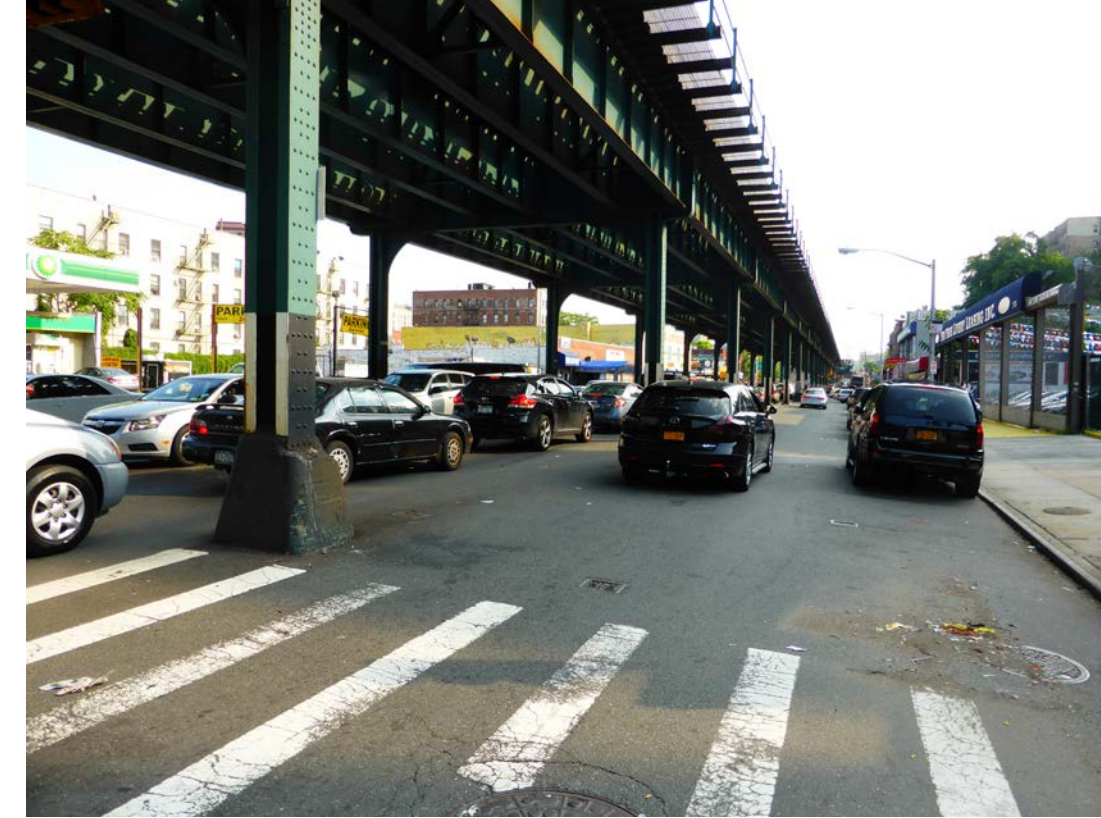
Dark, unattractive, vehicles swerving in & out between columns
