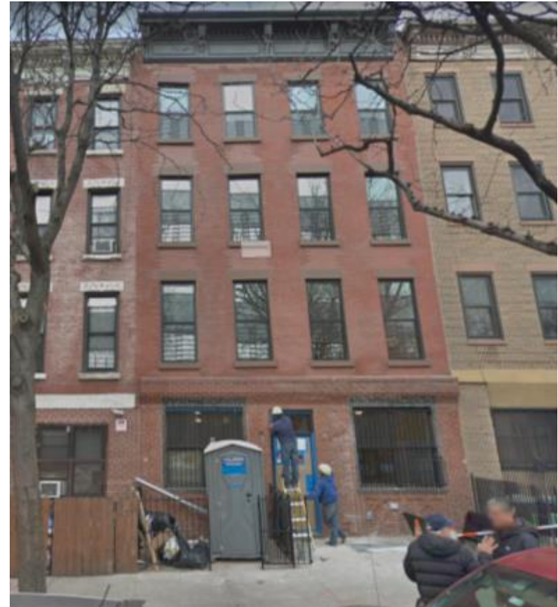
677 Union Street was renovated and refinanced in 2017 by owner Fifth Avenue Committee through HPD's LIHTC Year 15 program.
