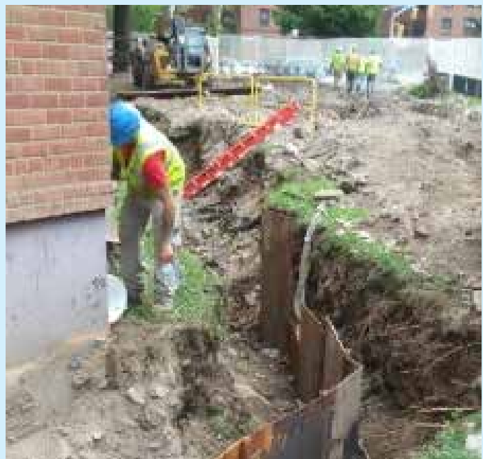
Passive impermeable barriers below grade stop water infiltration and protect building foundations. This photo shows flexible liners being installed below grade at Wald Houses in Manhattan. Credit: NYCHA
