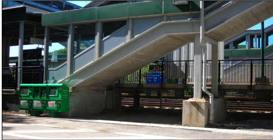
Existing Spuyten Duyvil station with available space beneath the stairs for bicycle parking
