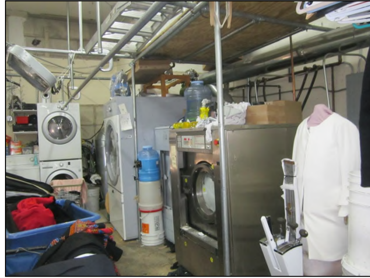
Photograph 26. Washing machines in the dry cleaner space.
