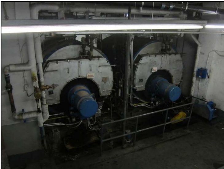
Photograph 3. Boilers in the basement of 470 Lenox Terrace.
