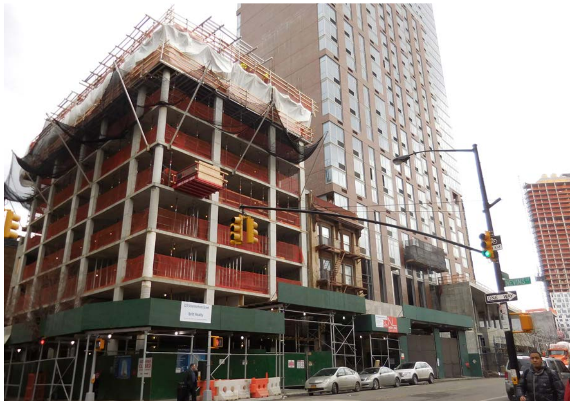
1. View East at Schermerhorn St. and Nevins St. intersection. Foreground shows two residential high-rises under construction. Photograph taken on: 02/10/2016
