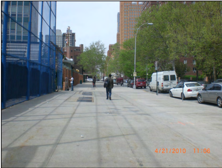
Photograph 5. Electrical transformer vaults in the northern Property sidewalk and a LIU dormitory (west-adjacent to the athletic field), looking west along Willoughby Street.
