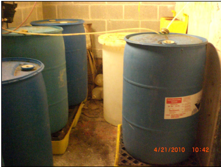
Photograph 9. Hydrochloric acid storage (for pool maintenance) in the basement of the athletic center.
