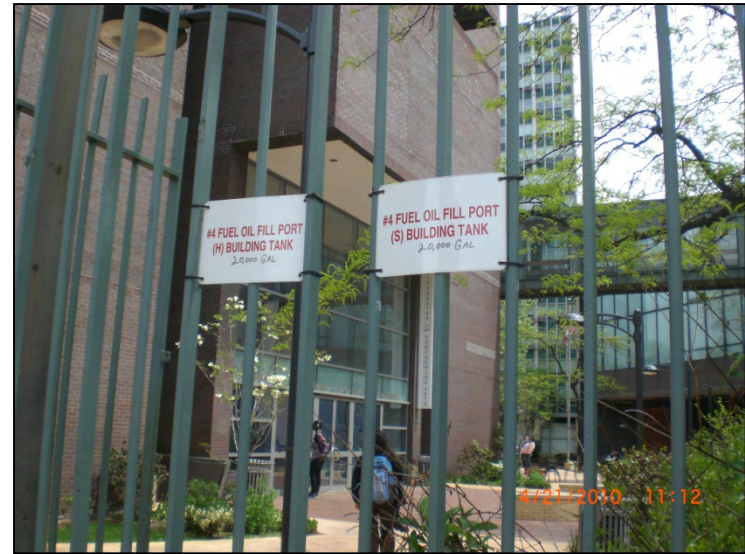
Photograph 10. Signs over the fill ports for two, 20,000-gallon fuel oil tanks in the western portion of the campus, southwest of the Property.
