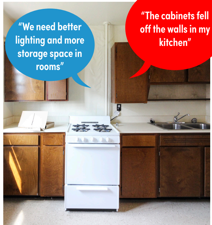
Residents noted that repairs and upgrades are needed in the kitchens. Cabinets are frequently broken, there is a lack of preparation surface, and appliances are dated.
