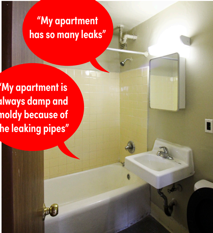
Residents stated that the current plumbing system is aged and frequently fails, flooding apartments, promoting mold growth, and leaving them unsafe for extended periods of time.
