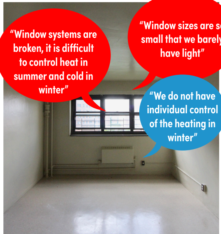
Residents expressed frustration in the lack of in-unit temperature control. Small and dirty windows restrict the amount of natural light, contributing to dim interior environments.
