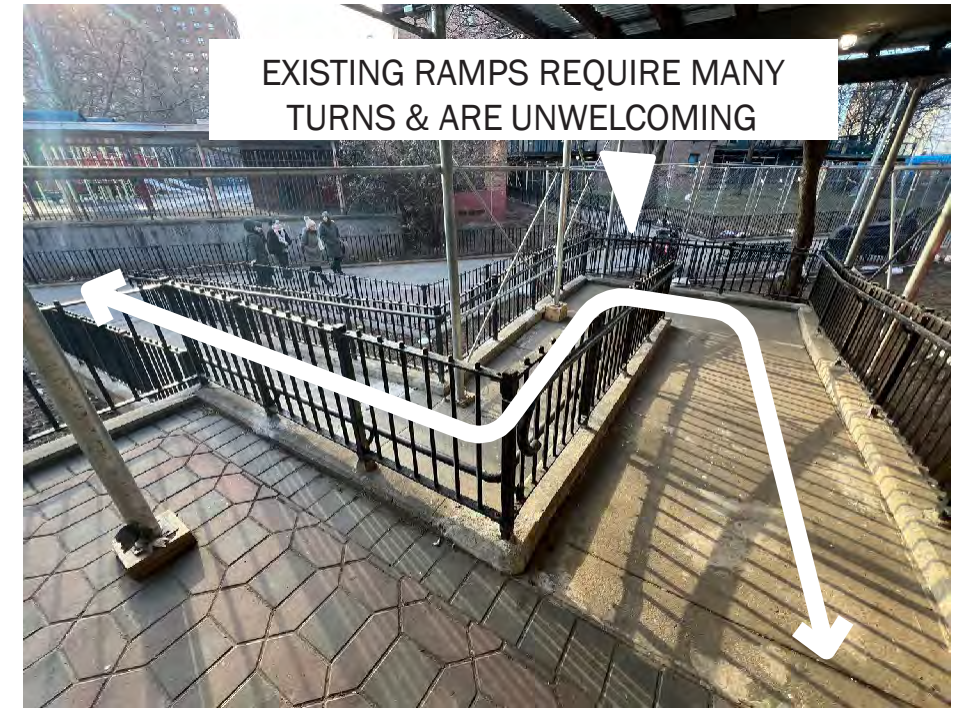
Existing ramps are dimly lit
