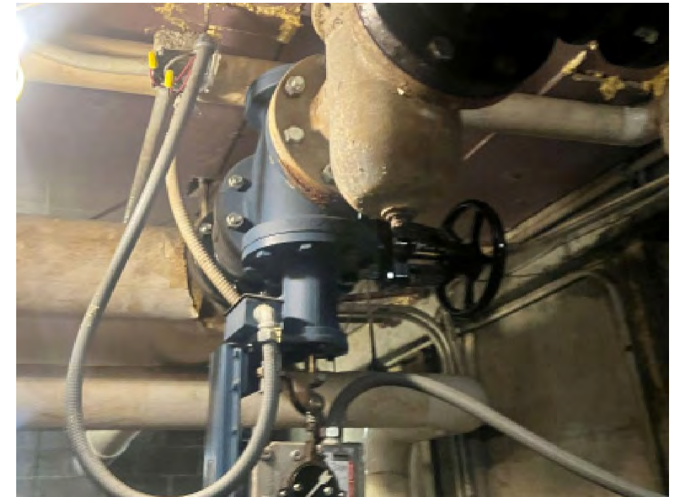
Zone control valves control the steam to each building, and are in good condition
