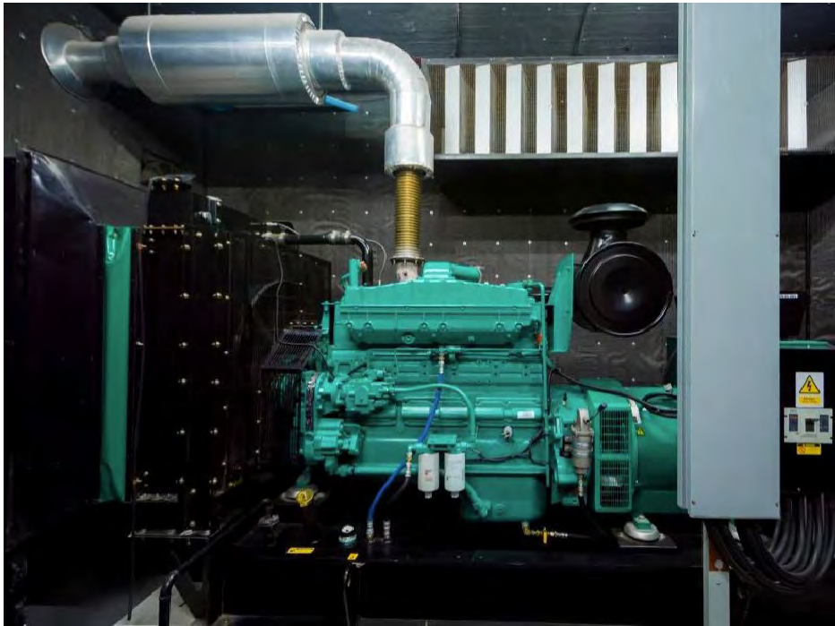
EMERGENCY ELECTRICAL GENERATOR
