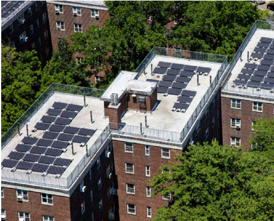
SOLAR PHOTOVOLTAIC ARRAY
