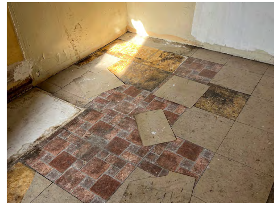
Multiple layers of damaged tile
