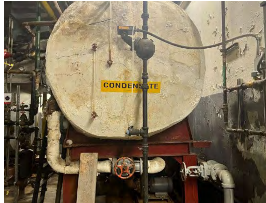
There is one 1,600 gallons capacity boiler feed tank
