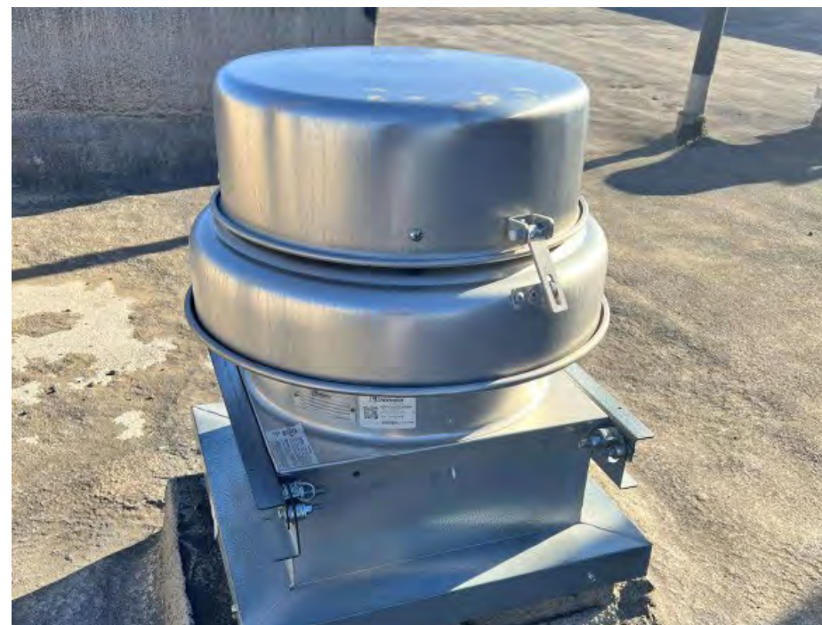
Exhaust fans are noted to be new and in good condition
