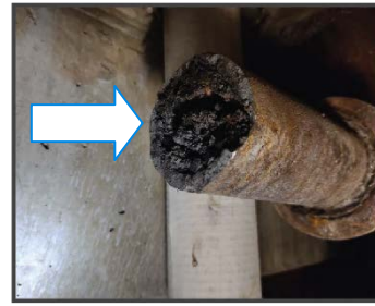
Interior surface of waste branch line (cast iron section) at Howard with significant sediment/debris accumulation
