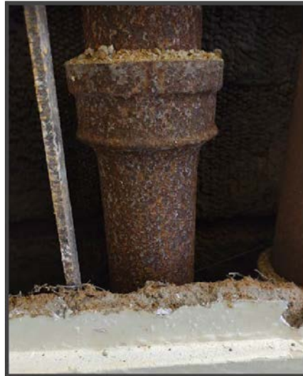
Waste riser at Howard considered to be in poor condition based on exterior physical appearance (excessive exterior corrosion)
