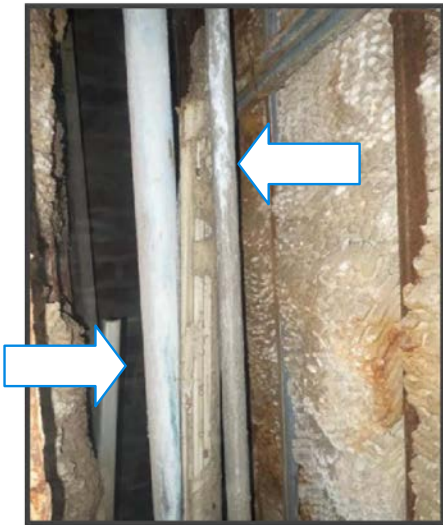
Domestic water risers at Queensbridge North displaying possible chemical reaction or de-zincification of the brass, suggesting that the pipes are at the end of their service life and may be subject to failure in the near term
