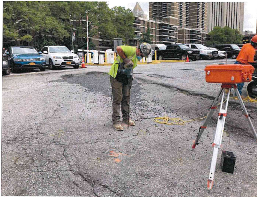
Photo 1: AARCO advancing a handheld hammer drill into a suspected void space (facing west)
