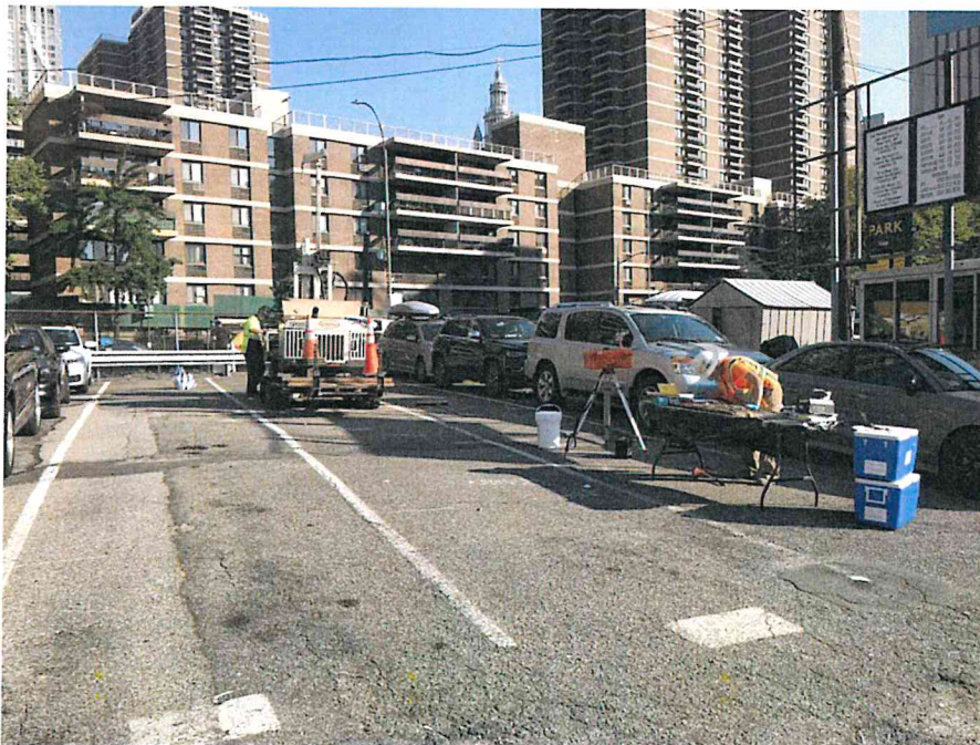
Photo 4: AARCO advancing soil boring SB4N1 and Langan sampling soil in the northern part of the site (facing north)
