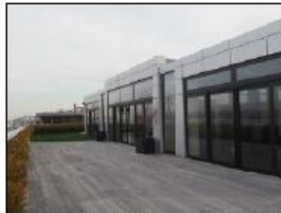
27 PENTHOUSE WEST FACADE - GENERAL VIEW FROM TERRACE, LOOKING NORTH NOT TO SCALE
