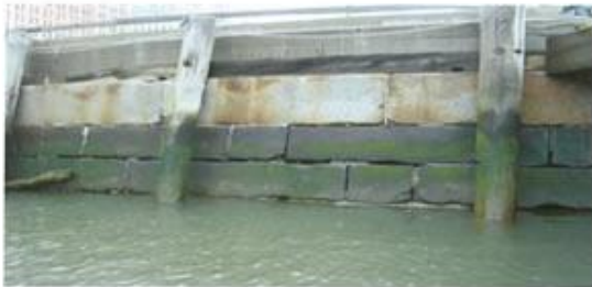
PHOTO 2 - North bulkhead wall concrete block with stone block cap up to 100% missing mortar in joints looking east.
