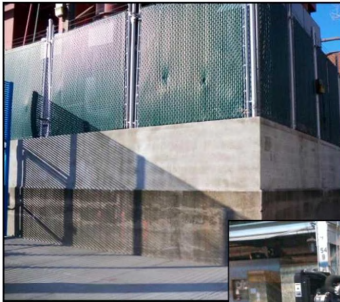
East River S/S – Raised Walls
