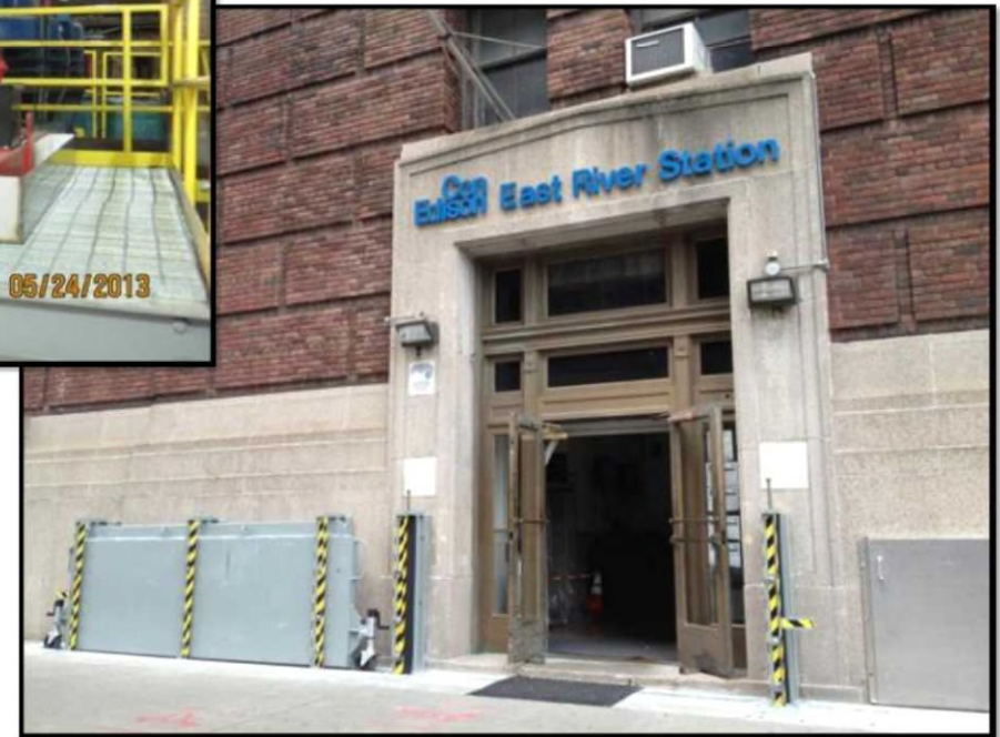
East River – Sliding Flood Door
