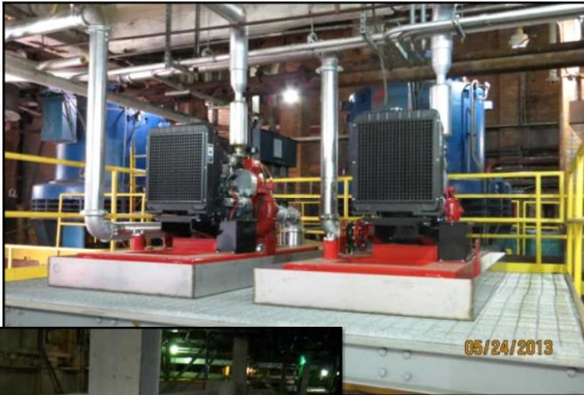
East River – Diesel Driven Pumps
