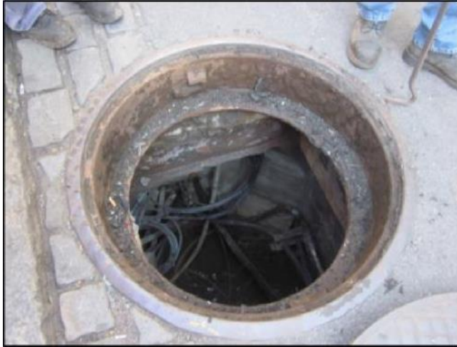
11 MANHOLES WITH DUCTS AND CABLES
