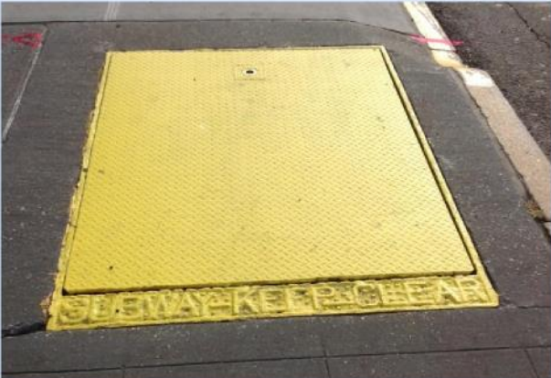
Emergency Egress & Access Hatches
