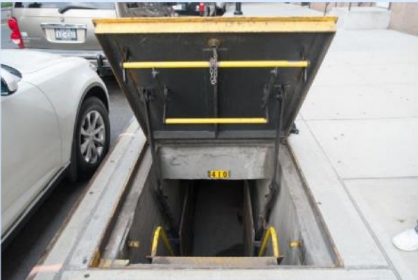
Water Tight Hatches
