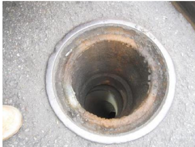
16 10 INCH PULLING MANHOLES
