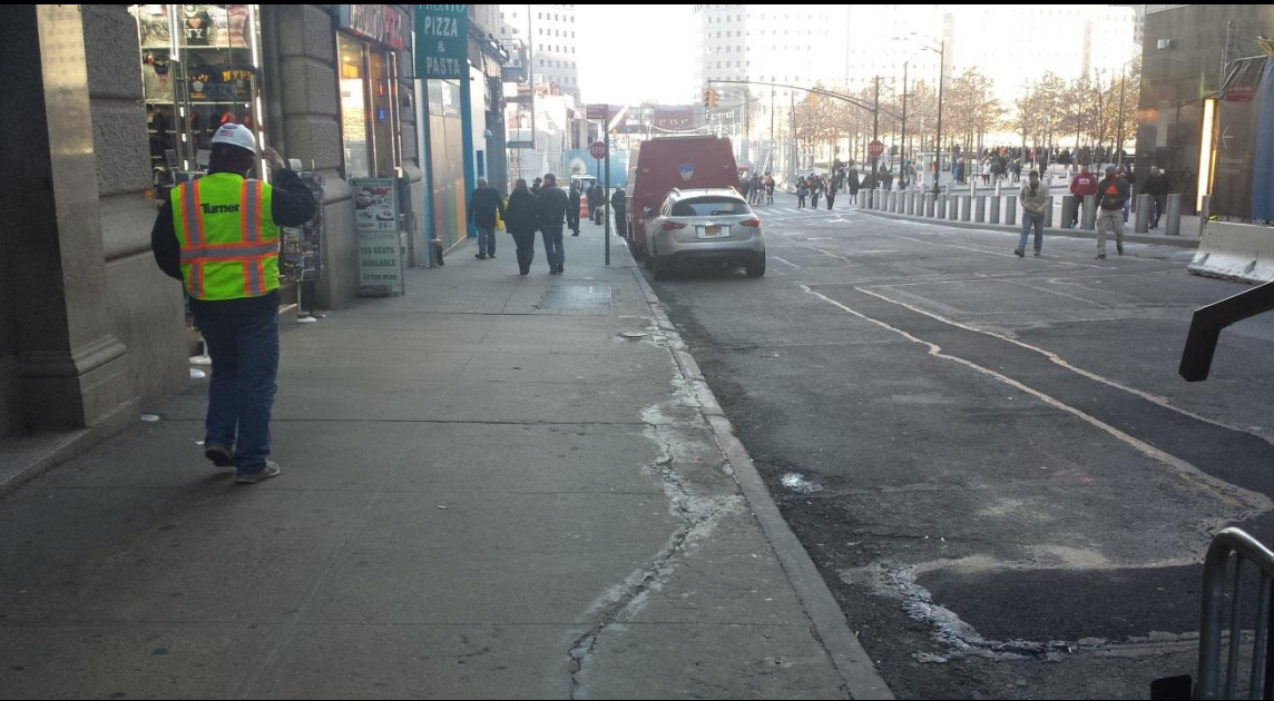
Liberty Street -- Removal of barricades on southern sidewalk beyond security clamshell and removal of hoist from 4 WTC (12/08/14)
