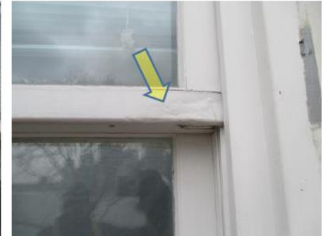
WOOD DECAY BEHIND PAINT -UNSAFE CONDITION-
