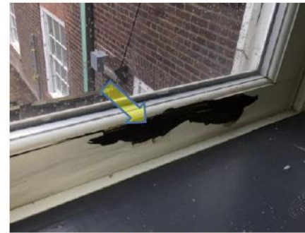
INTERIOR WOOD DECAY OF SASH FRAMING
