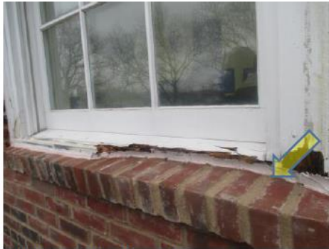
WOOD DECAY OF EXTERIOR SILLS
