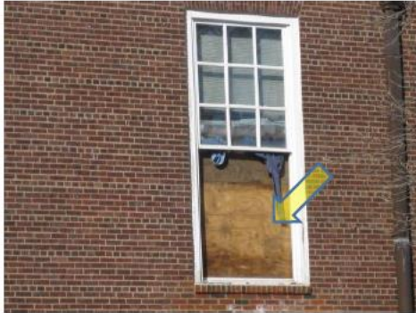
COLLAPSED WINDOW SASH DUE TO WOOD DECAY -UNSAFE CONDITION-
