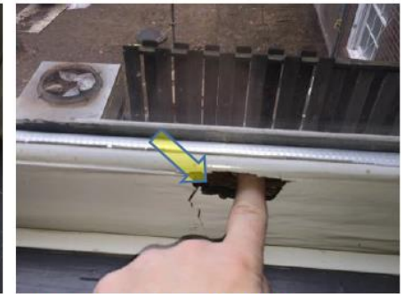
INTERIOR WOOD DECAY OF SASH FRAMING
