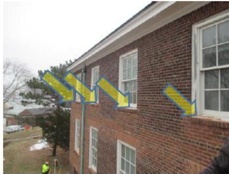
WOOD DECAY OF EXTERIOR SILLS
