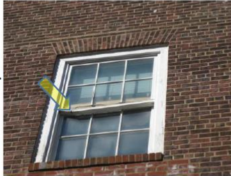
BROKEN WINDOW SASH DUE TO WOOD DECAY. -UNSAFE CONDITION-
