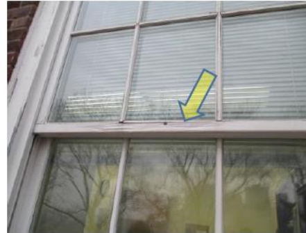
WOOD DECAY BEHIND PAINT -UNSAFE CONDITION-
