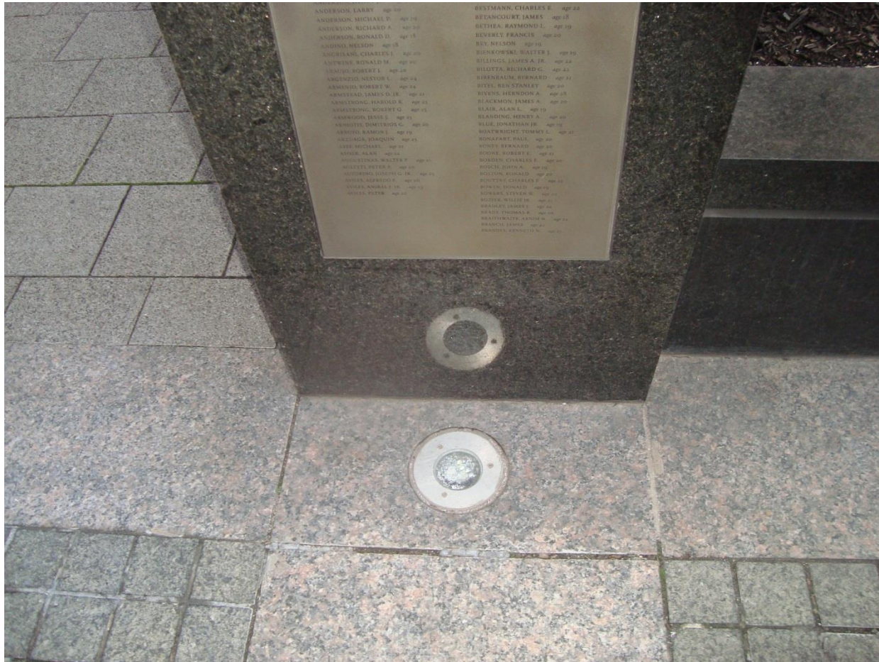
Ground Plane Lighting (to be removed and replaced with granite to match exist.)
