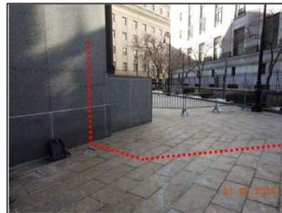
PHOTO #10 - EXISTING BLUESTONE PAVERS ARE INSTALLED POSSIBLY OVER UNEXCAVATED GRADE IN THIS AREA. FENCE WILL BE HELD 24" AWAY FROM STAIR SO THE FENCE CANNOT BE SCALED FROM STAIR.
