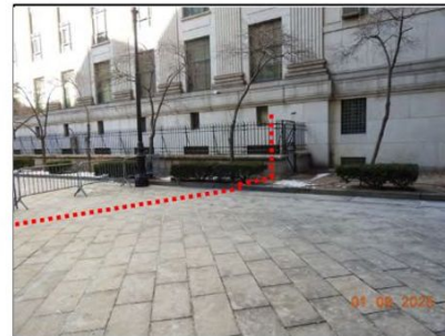
PHOTO #11 - EXISTING BLUESTONE PAVERS ARE INSTALLED POSSIBLY OVER UNEXCAVATED GRADE IN THIS AREA. THIS WILL NEED TO BE CONFIRMED.
