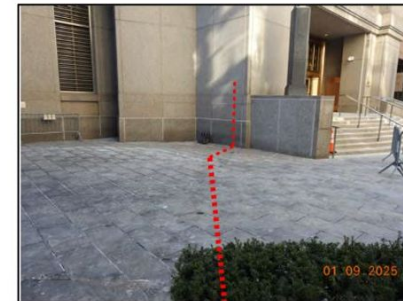
PHOTO #9 - EXISTING BLUESTONE PAVERS ARE INSTALLED POSSIBLY OVER UNEXCAVATED GRADE IN THIS AREA.
