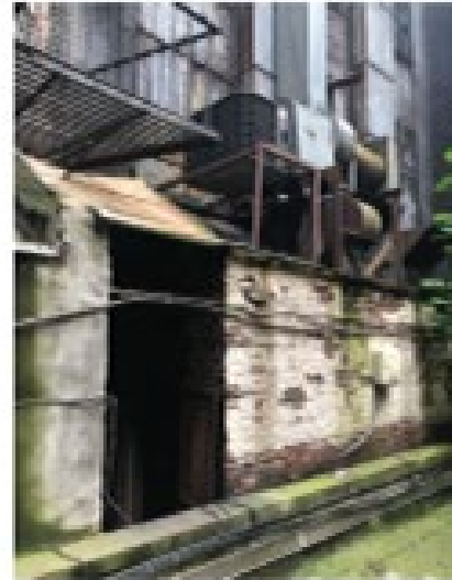
Crack condition at No.62 rear yard
