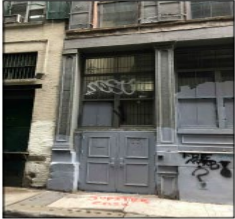
01 PHOTO AT SOUTHERN—MOST EGRESS DOOR
