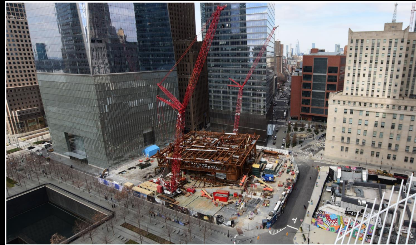
March 2020: Progress view of steel erection – now at Play level. View from southeast.
