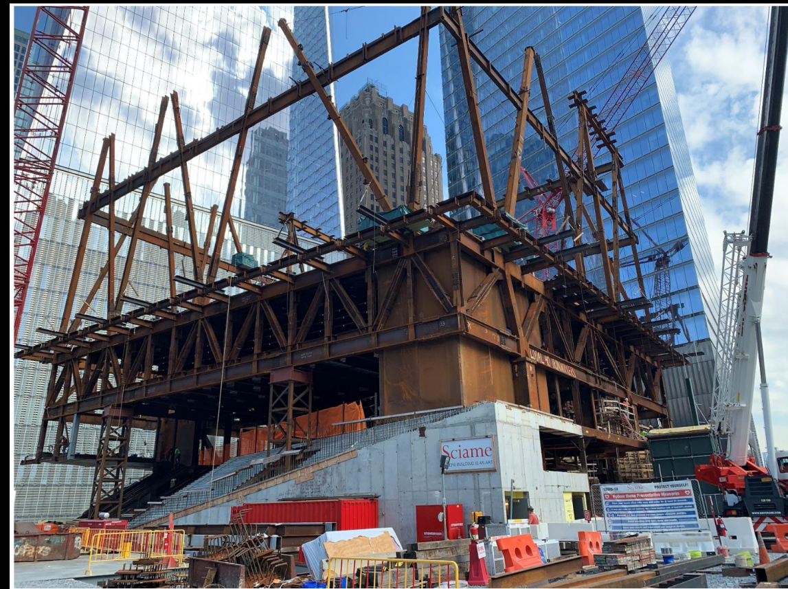
July 2020: Steel trusses begin to rise after COVID-19 delay. View from southeast.
