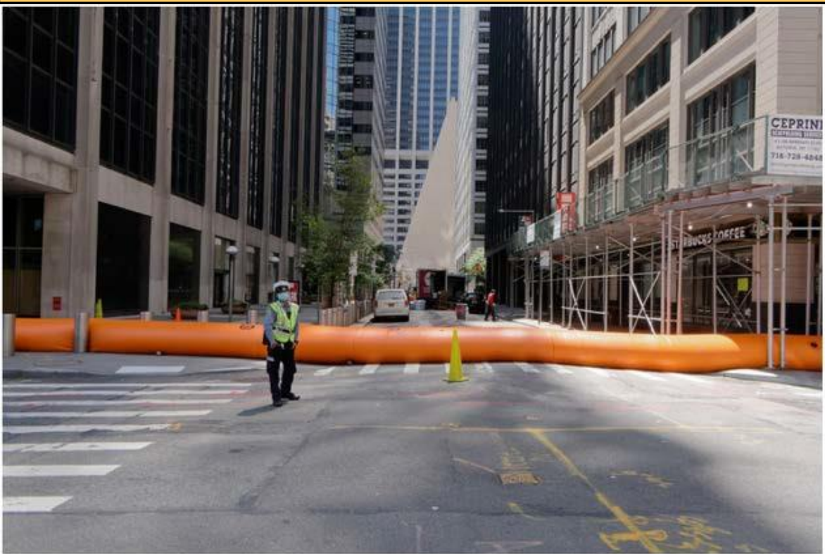
A Tiger Dam crosses Front Street along Wall, linked to a continuous set of barriers from Catherine Slip to Water Street. Photo: Carl Glassman/Tribeca Trib
