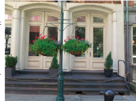
EXISTING PAINTED DIAMOND PLATE STEEL STAIRS, SECTIONS MISSING AT BASE
