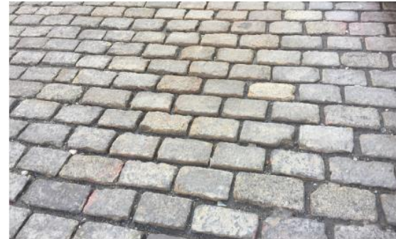
Grout not flush with surface, joints too wide
