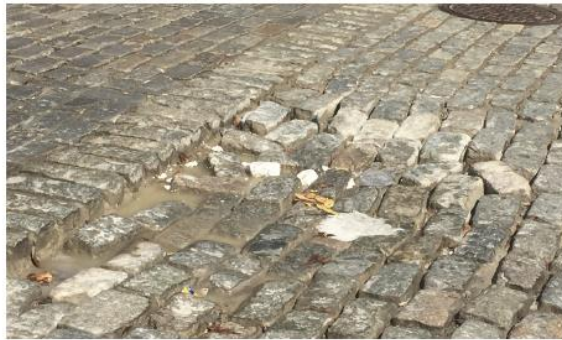
Collapsed concrete base, deteriorating grout, stones unaligned
