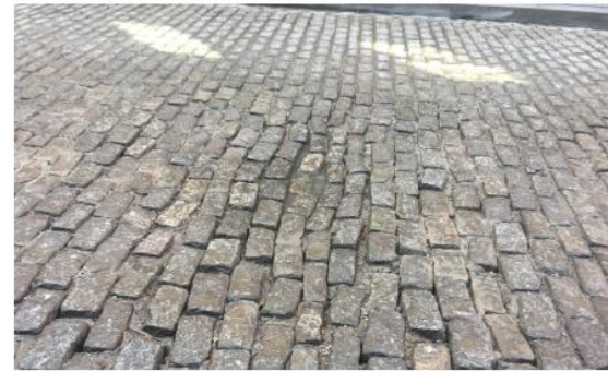
Deteriorating grout, stones unaligned, joints too wide
