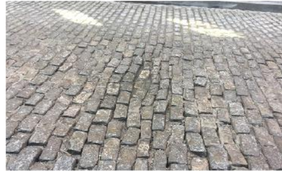
Deteriorating grout, stones unaligned, joints too wide
