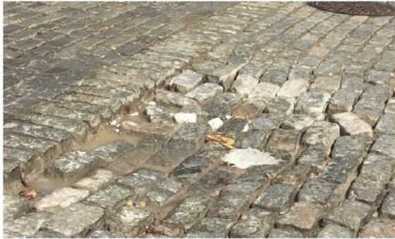
Collapsed concrete base, deteriorating grout, stones unaligned
