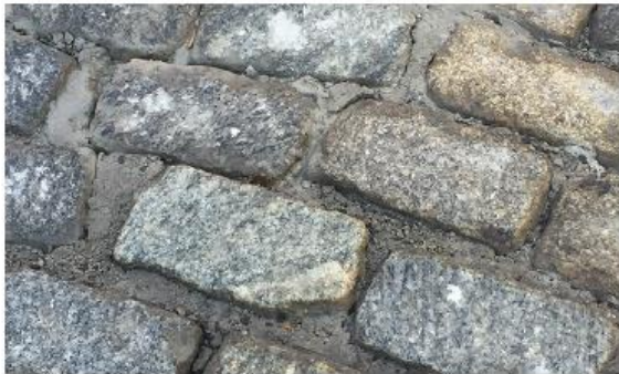
Grout not flush with surface, grout poorly maintained, joints too wide
