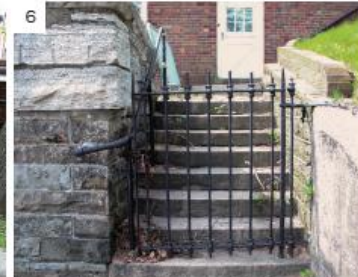
6 (2018) View of cast iron gate and pipe hand rail at upper wall
