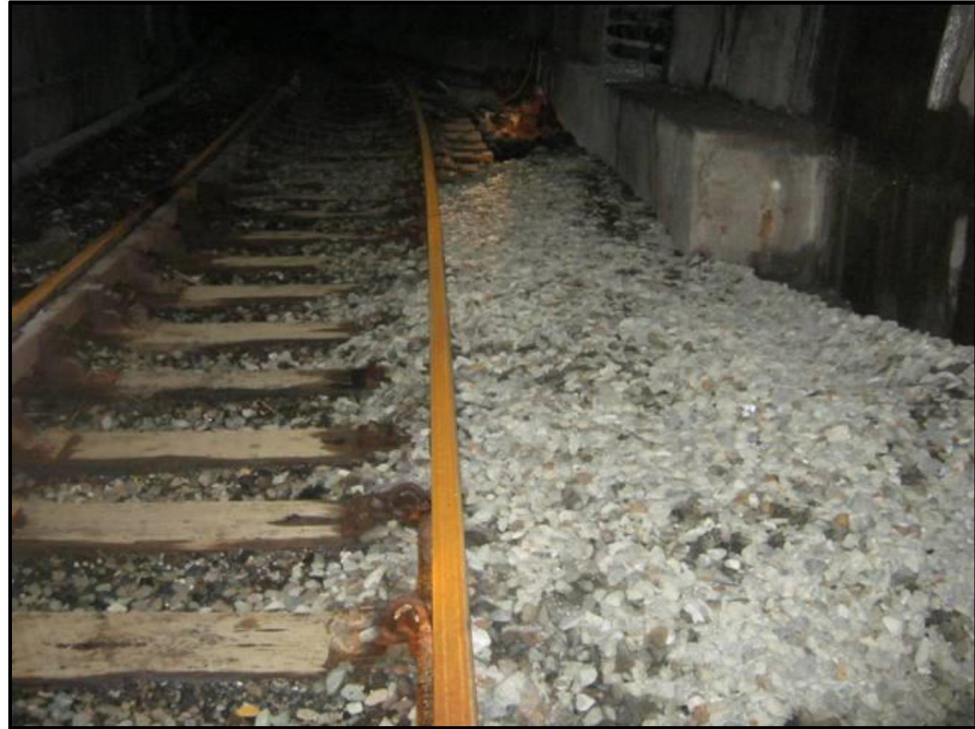
Corroded rail and fouled ballast in tunnel (11/3/2012)
