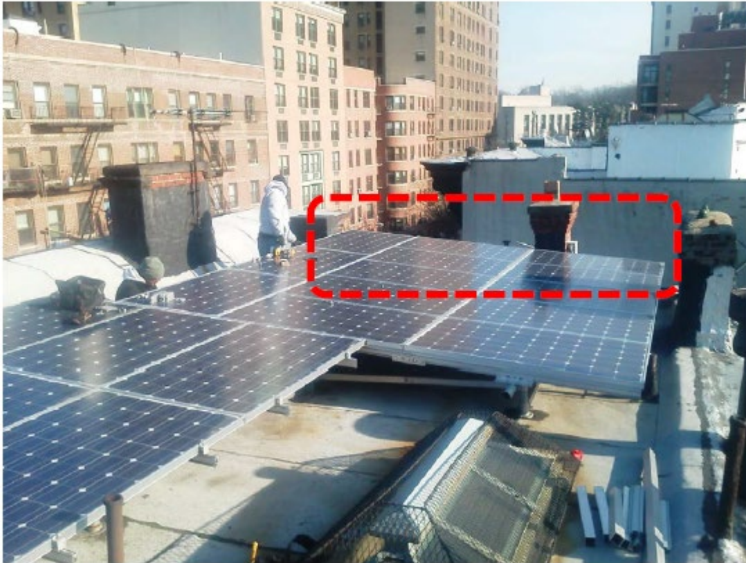
Figure 3: Solar panel installation “A” as seen looking towards the rear of the roof where visible from the street.
