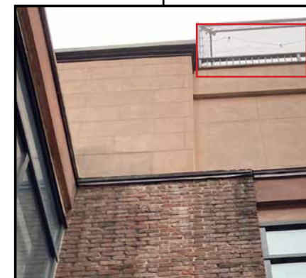
Light Fixtures and Mounting B
