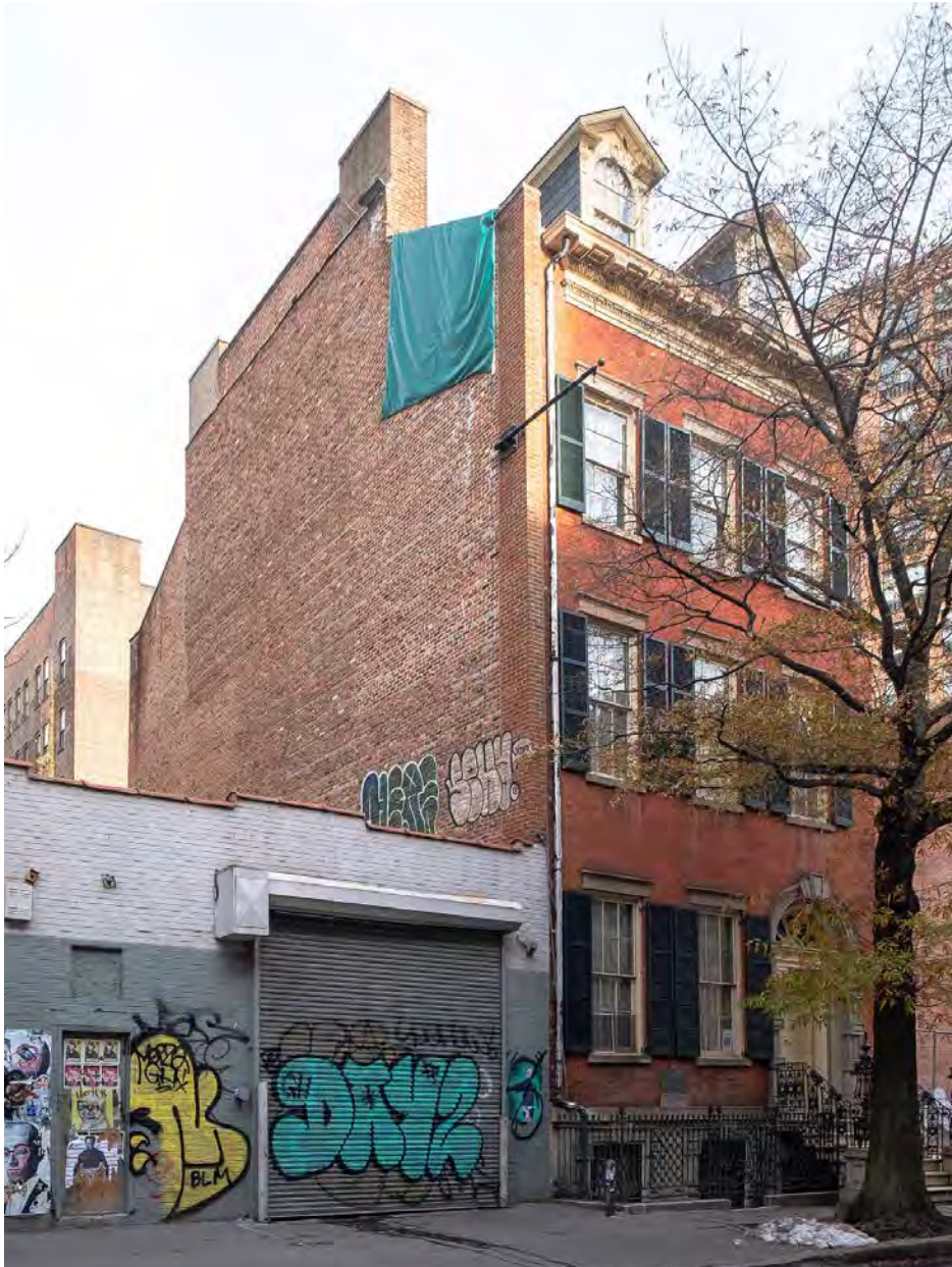
CURRENT LOT LINE WALL CONDITION
