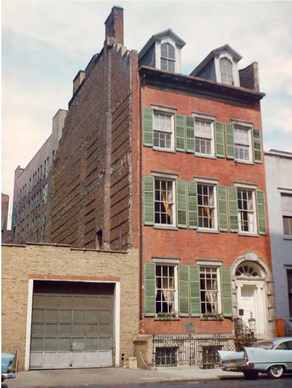
1960'S LOT LINE WALL CONDITION
