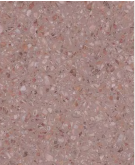
Precast Window Sills at East Facade
