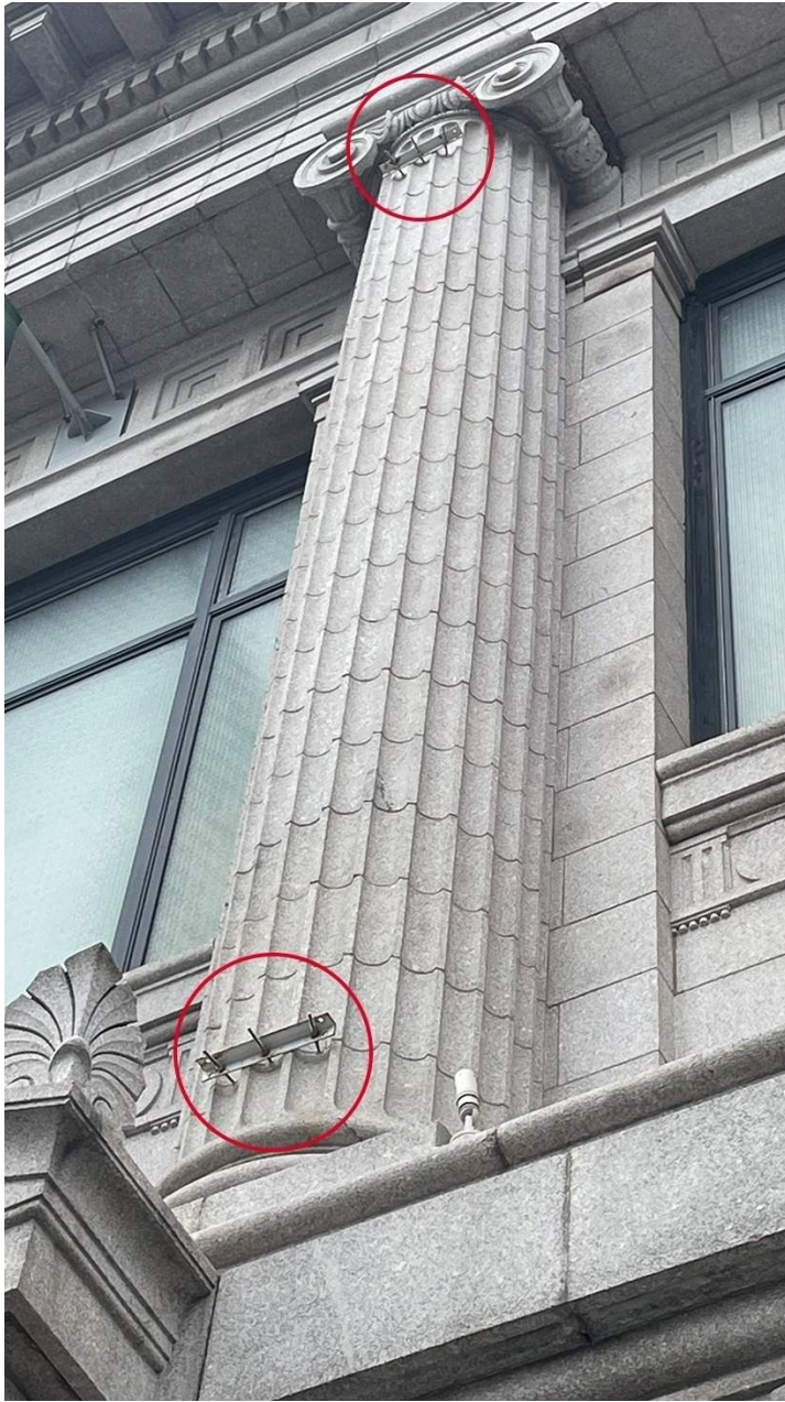
EXISTING BRACKET AT CENTER COLUMN TO REMAIN
