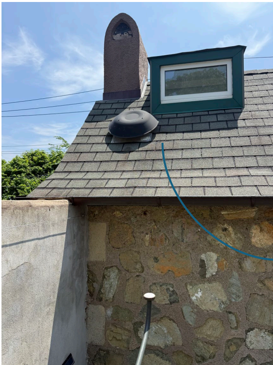
Current exhaust located on roof in kitchen, mushroom type, highly visible.
