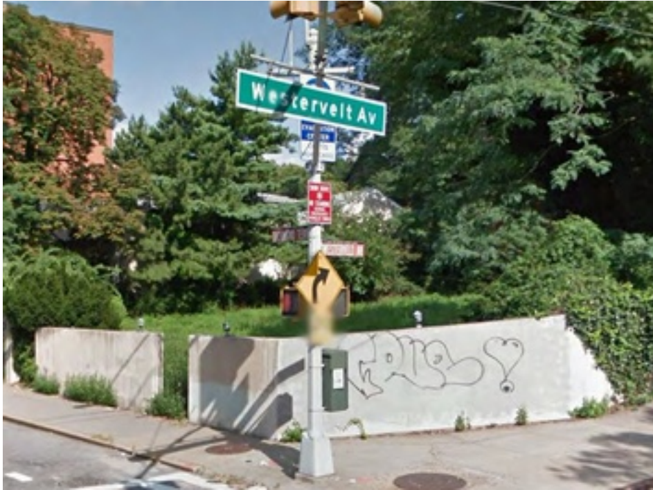
2012: exposed stucco perimeter wall with graffiti.
