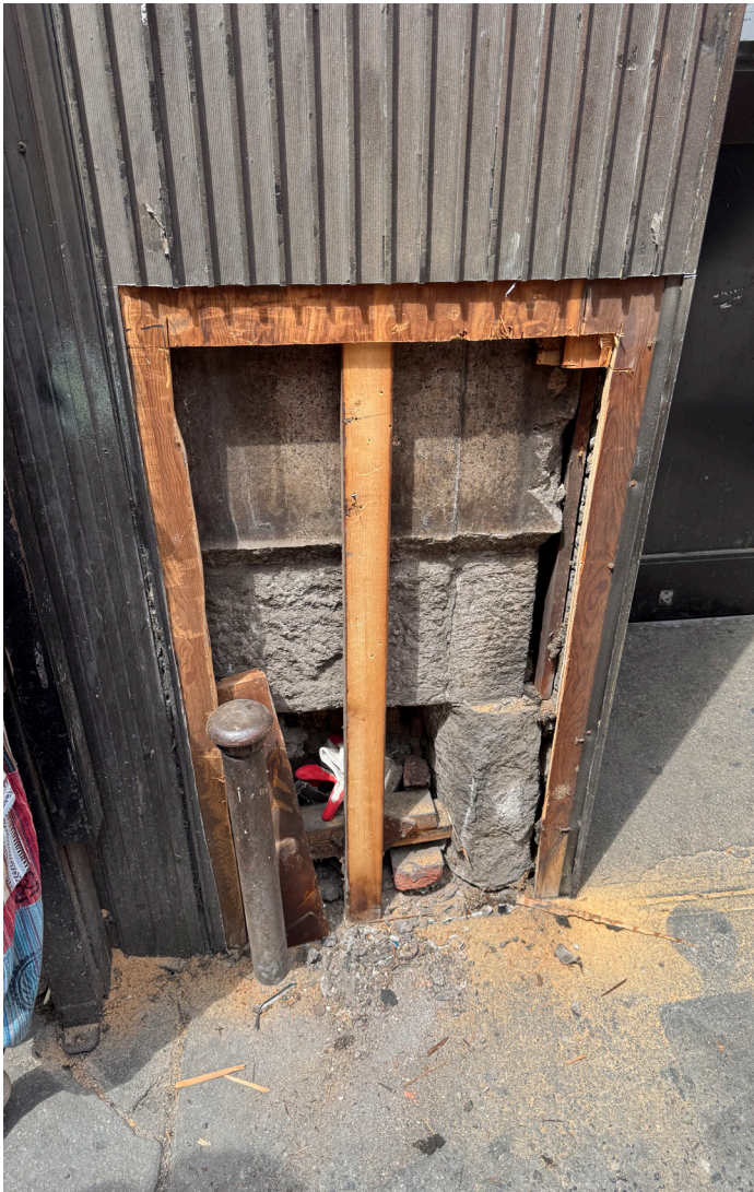
2026, Storefront - Base pier at Broadway
