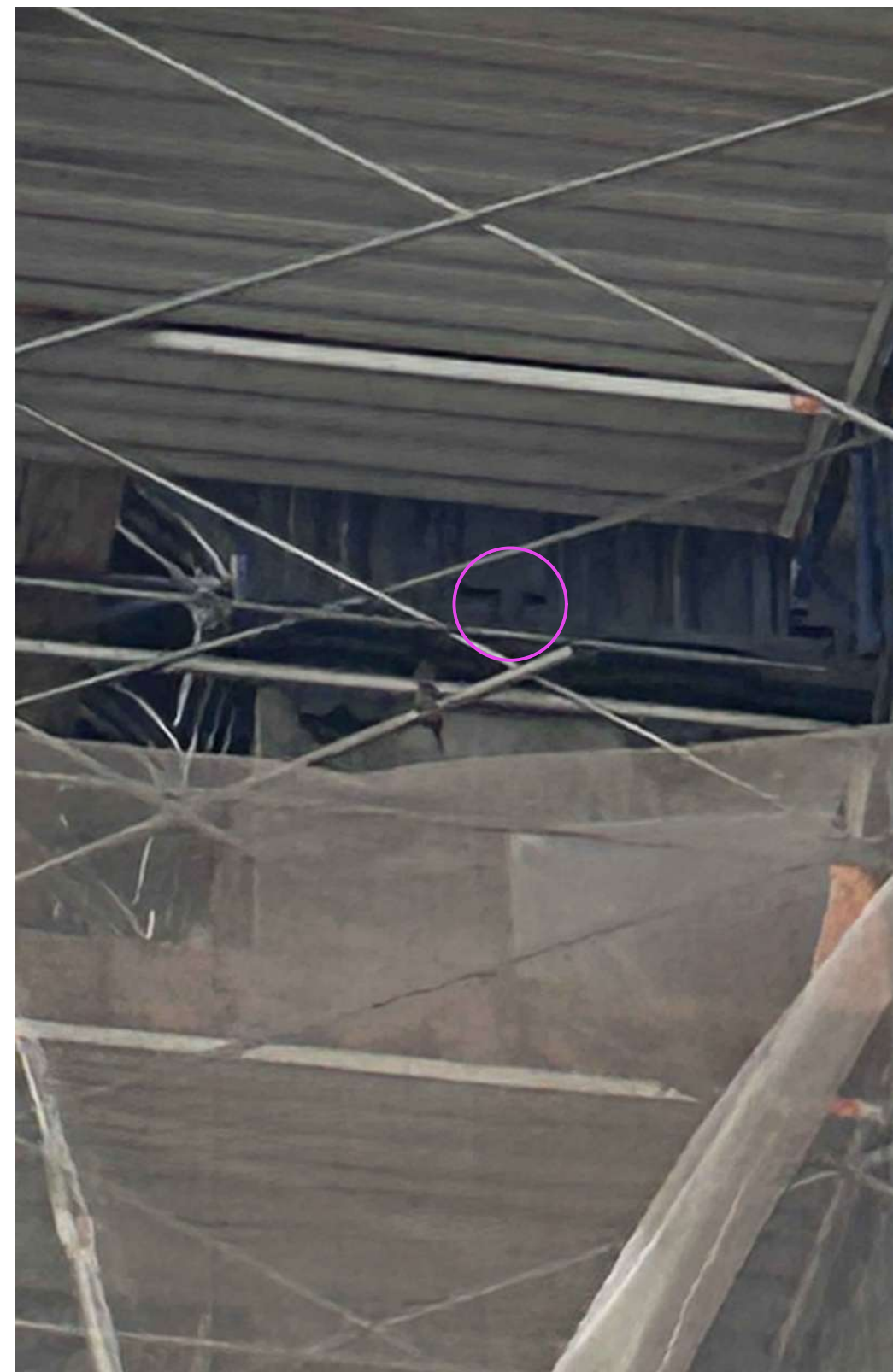
PHOTO 9. POINT D. CLOSE-UP PHOTO OF BLACK FIXTURE @ TOP CORNICE
