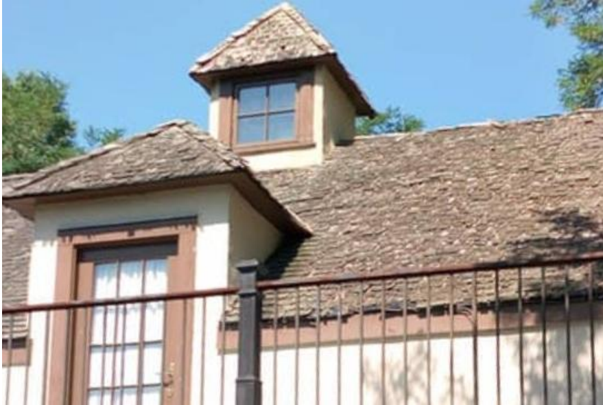
Rotting wood shingle roof. (Cyclopedia 2018)
