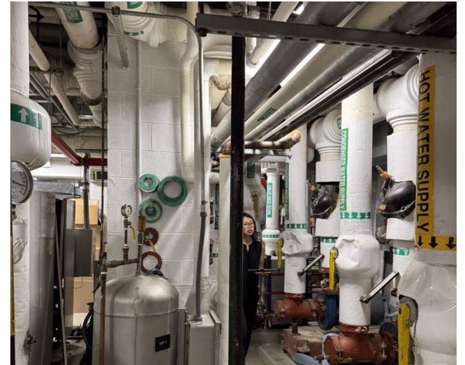
Existing Mechanical Room at Mansion
