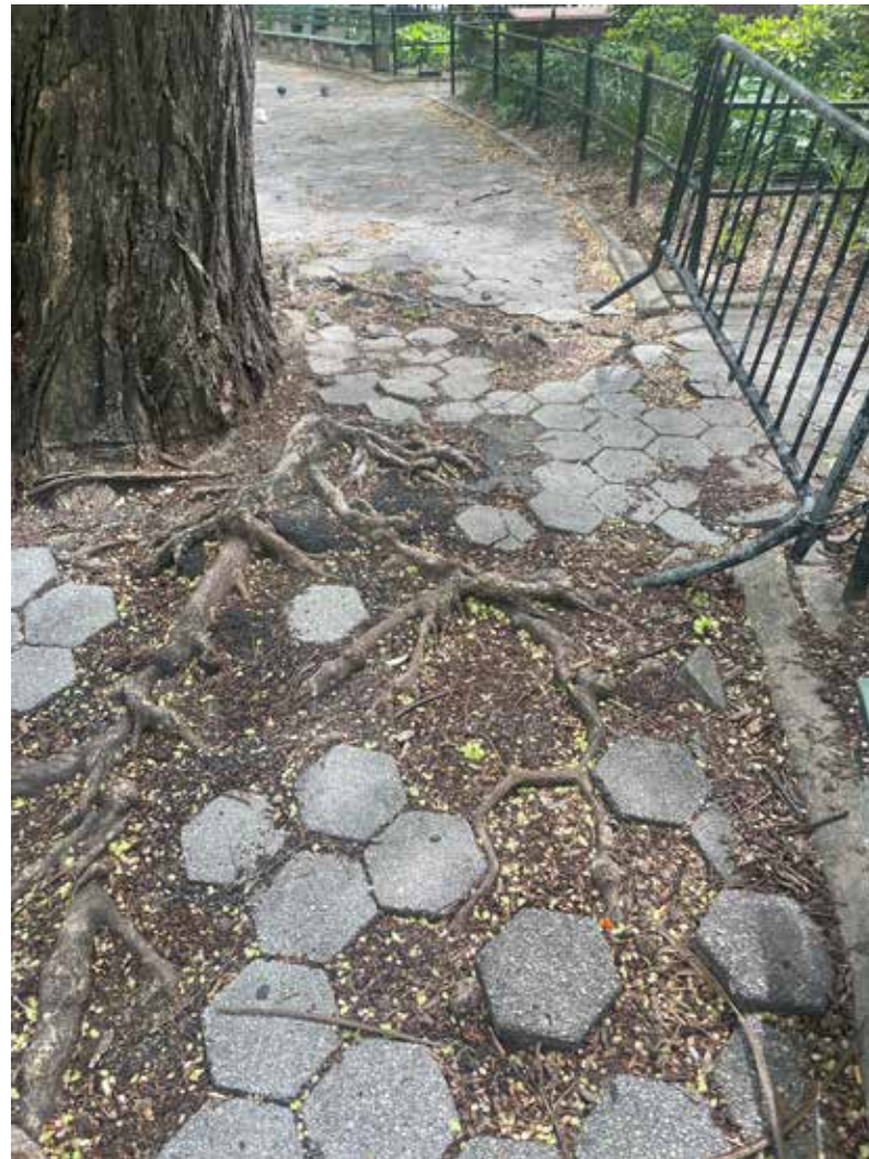
2 - Elm tree roots heaving and safety barrier in front of Men's entrance to PRB
