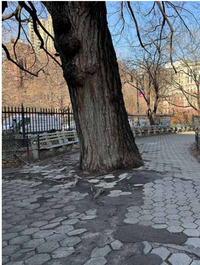
1 - Elm tree roots heaving and asphalt patches
