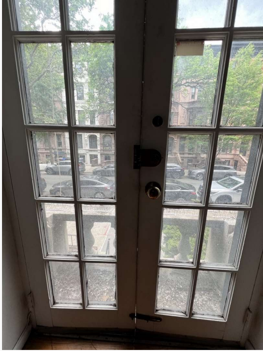
Interior view of existing balcony door — deteriorated glazing seals
