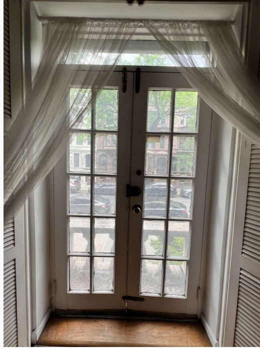
Interior view — multiple supplemental locking devices visible along center stile
