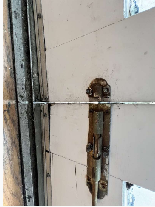
Close-up: rusted bolt lock at base — one of five locks added to keep door secured
