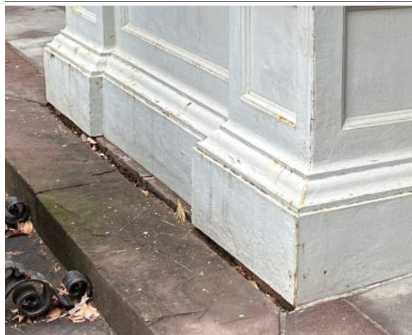
A17-2 - RESET DISPLACED CURBS AT PORTICO
