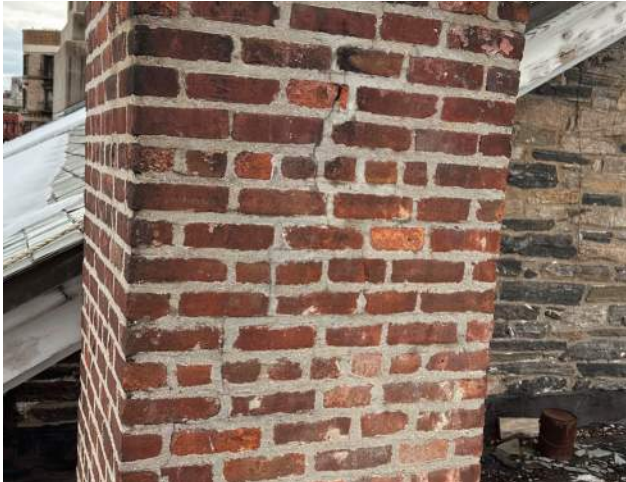
Chimney masonry shows cracked bricks and loose mortar.
