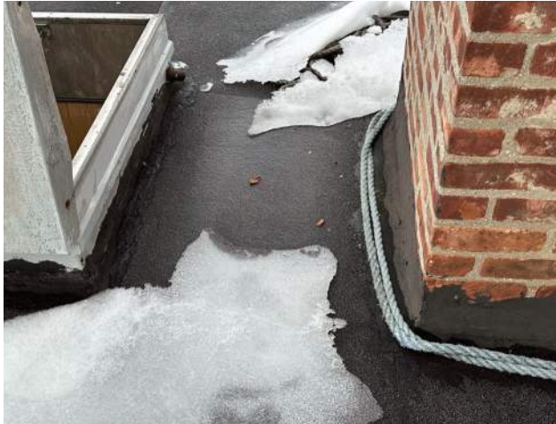
Typical base flashings on low-slope roofs are sheet membranes, but here are only applied tar.
