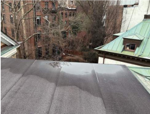
Open seams or other defects were not observed in the low slope membrane, however, water collected at edges and did not have scuppers to direct runoff.
