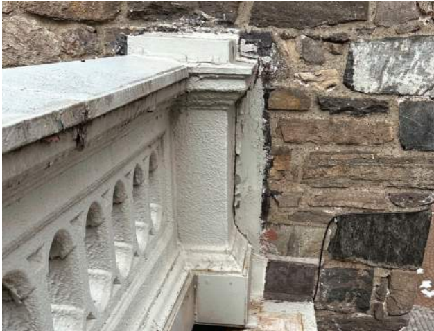
Iron posts of the parapet are flashed into the stone wall with galvanized sheet metal that has been overpainted. The end flashings are in poor condition.
