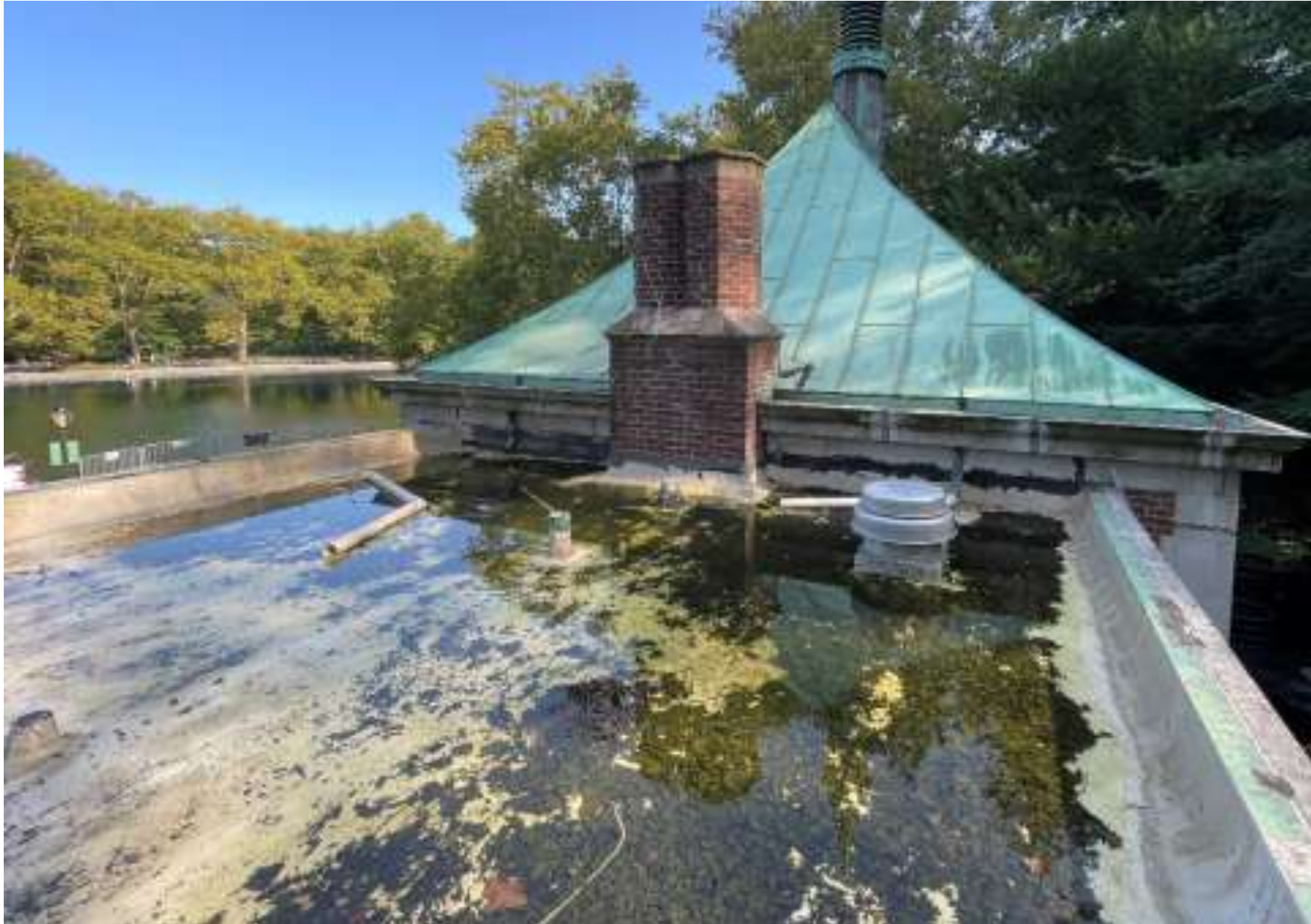
Overall view of the fluid-applied membrane roof assembly at the south wing
