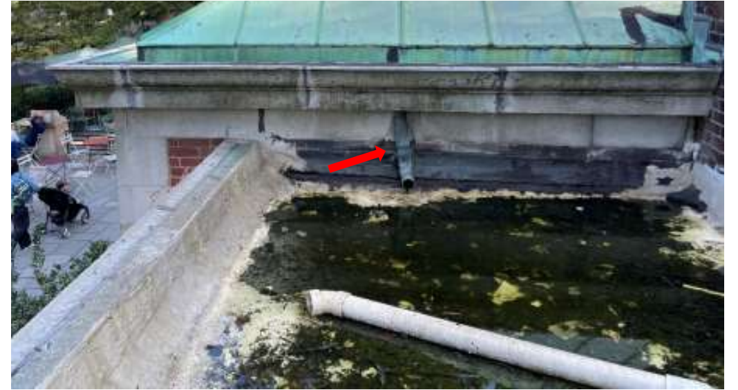
Damaged copper leader strap at the south wing flat roof
