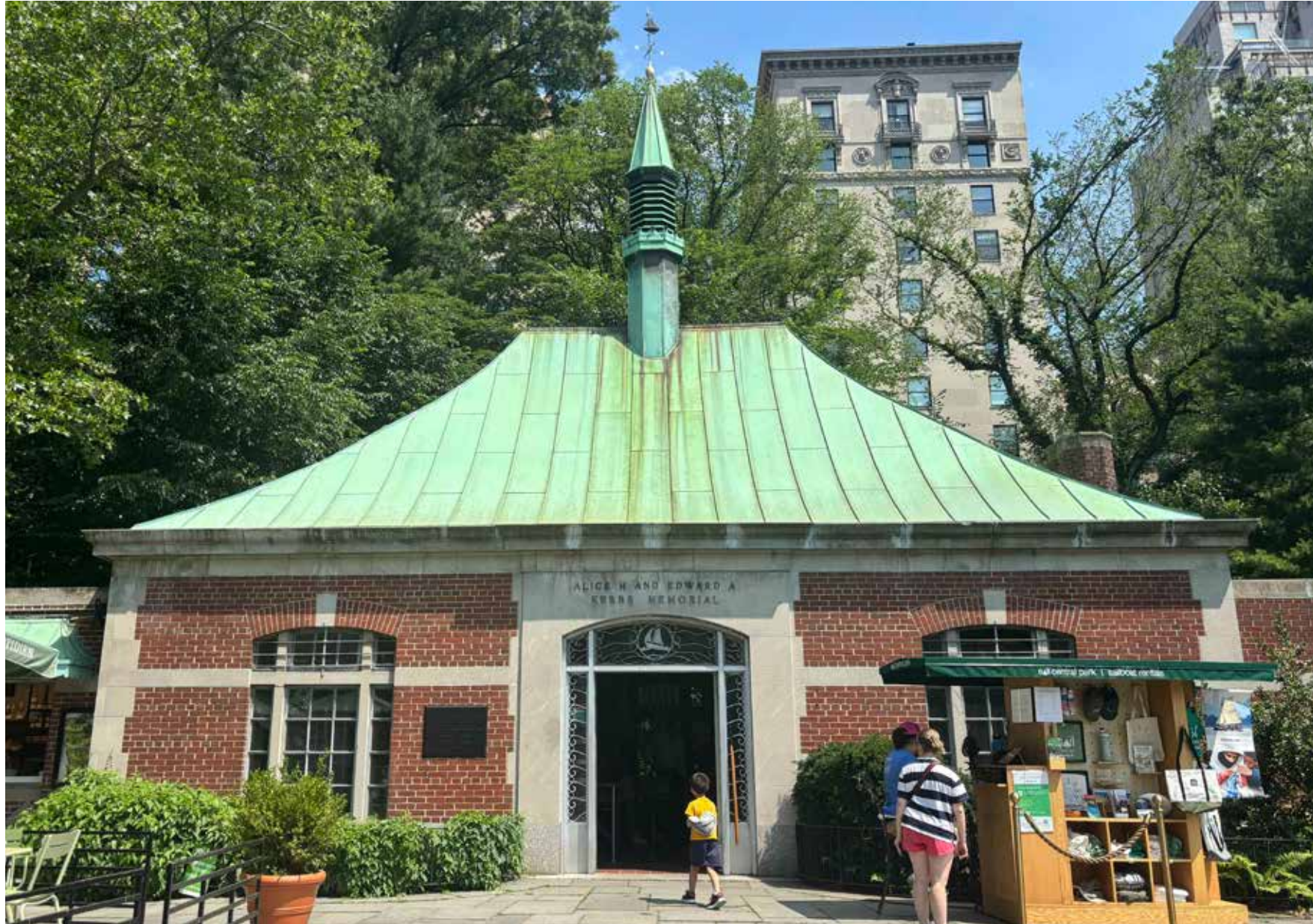
Existing copper roof staining
