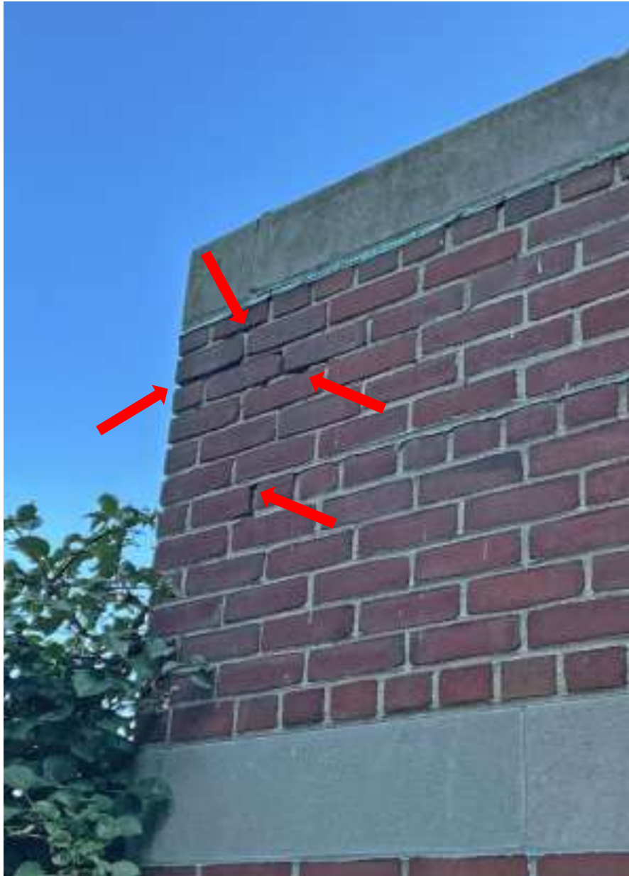
Open mortar joints and brick displacement
