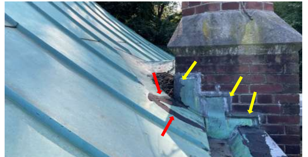
Tar applied at the Boathouse's copper cricket flashing seams (Red Arrows) and at the copper chimney step flashing (Yellow Arrows).
