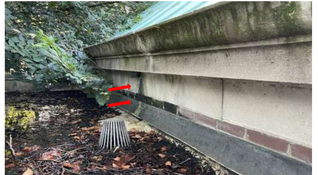
Missing leader section at the north wing flat roof
