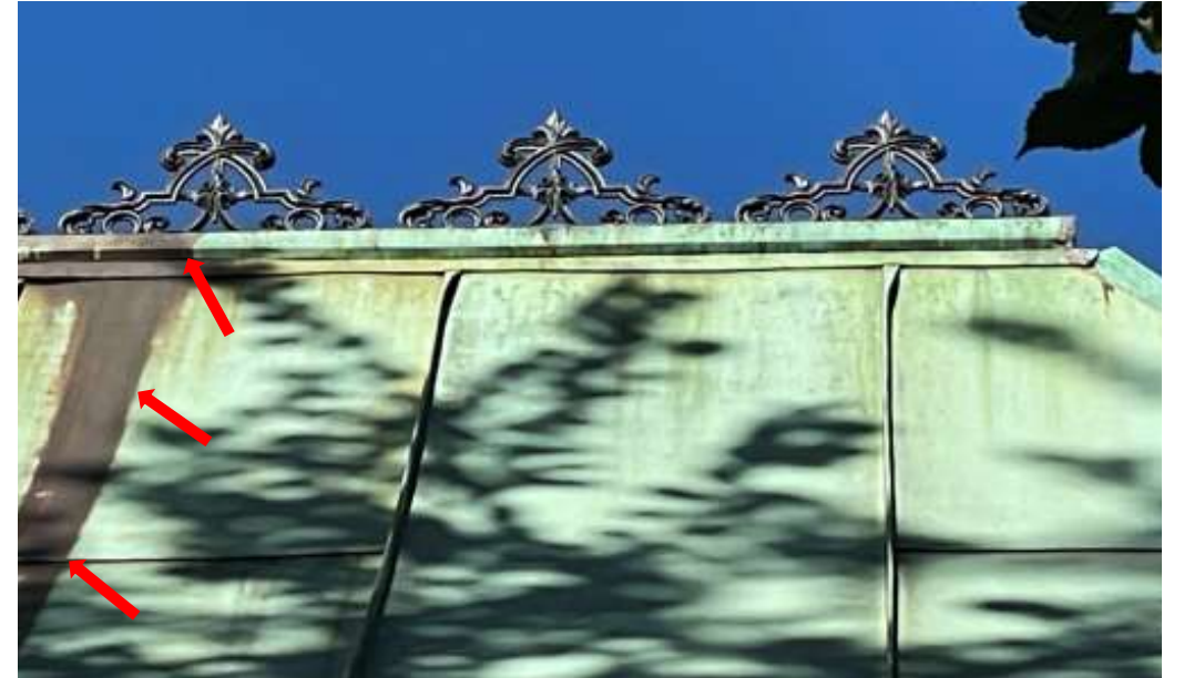
Metal Staining at the cast iron cresting and extending downward
