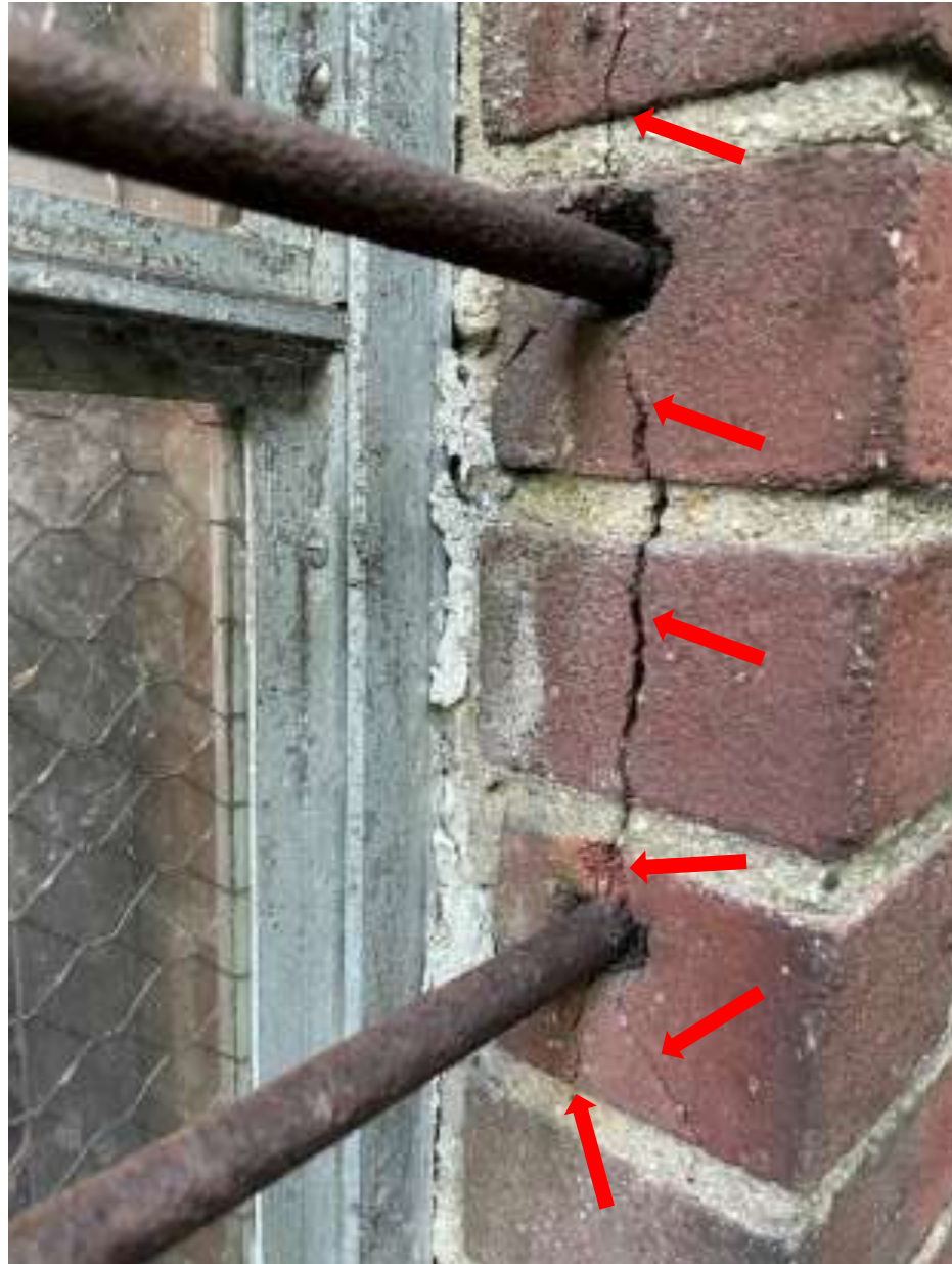
Cracked brick caused by corrosion of a steel window guard assembly
