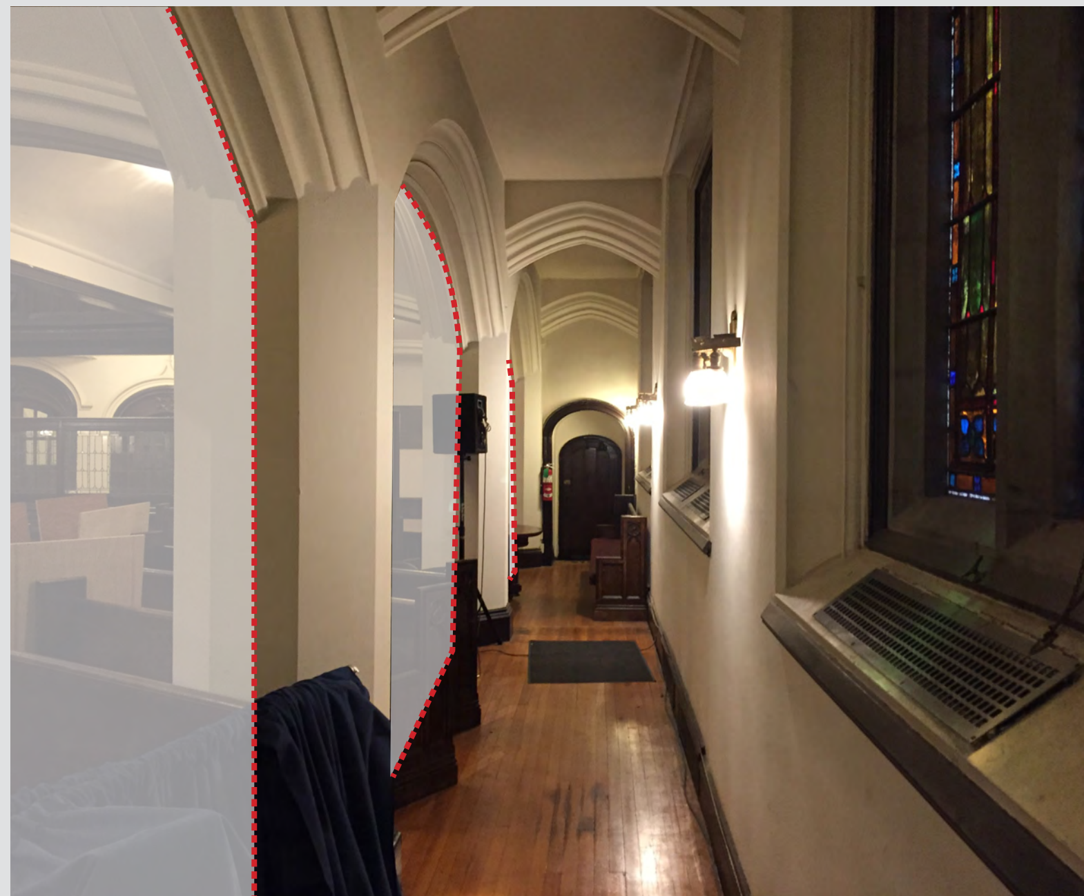
⑦ SOUTH CHURCH NAVE PASSAGE FROM THE TOWER DOOR TO THE PARISH HOUSE. DUE TO FREQUENT TRAFFIC, NAVE WOULD REQUIRE SEPARATION FROM THE MAIN CHURCH SPACE.
