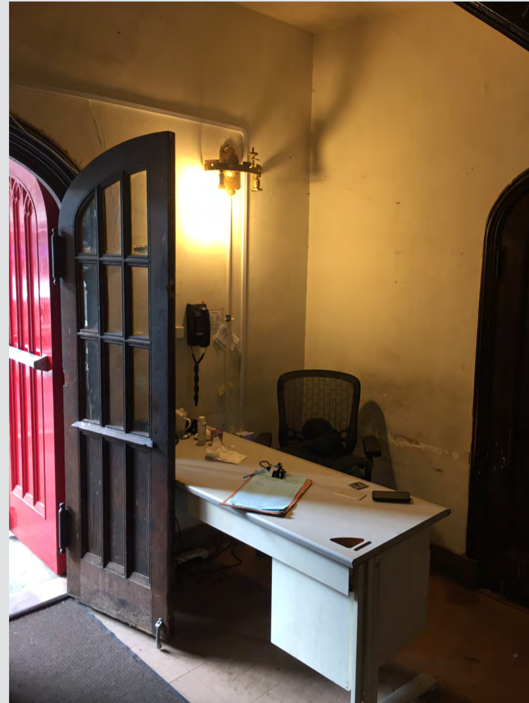
② INTERIOR CONDITIONS AT ENTRY TO THE TOWER AT WEST 114TH ST.
