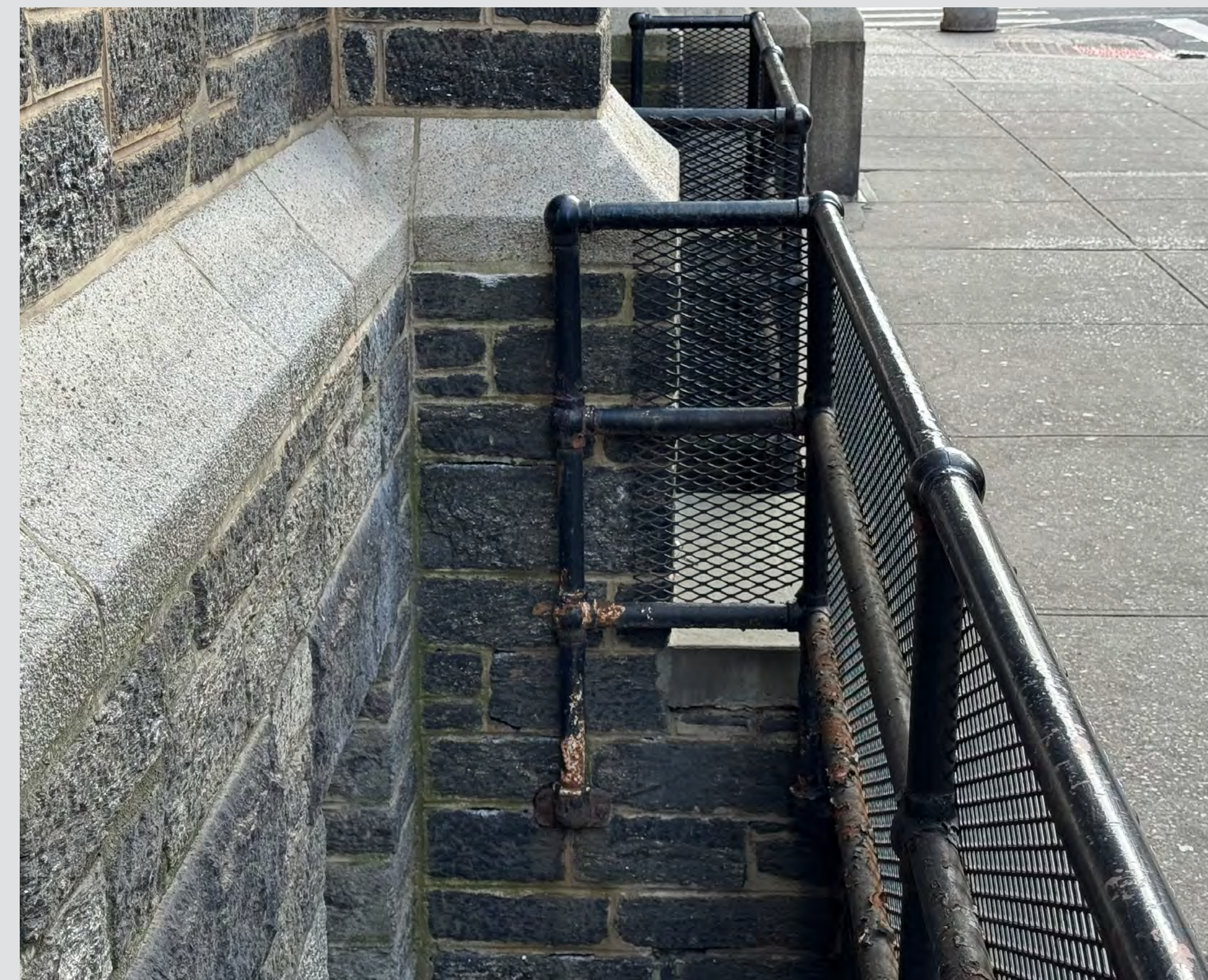
⑤ DETAIL OF TYPICAL WINDOW WELL NON-HISTORIC RAILING WITH ADDED IRON MESH.
