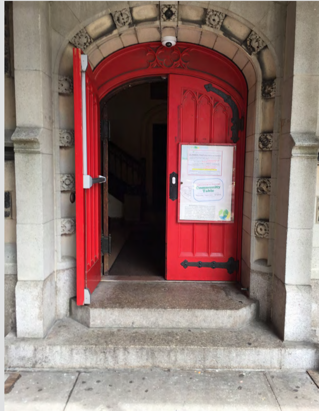
① ENTRY TO THE CHURCH'S TOWER AT WEST 114TH STREET. NOTE TWO ENTRY STEPS
