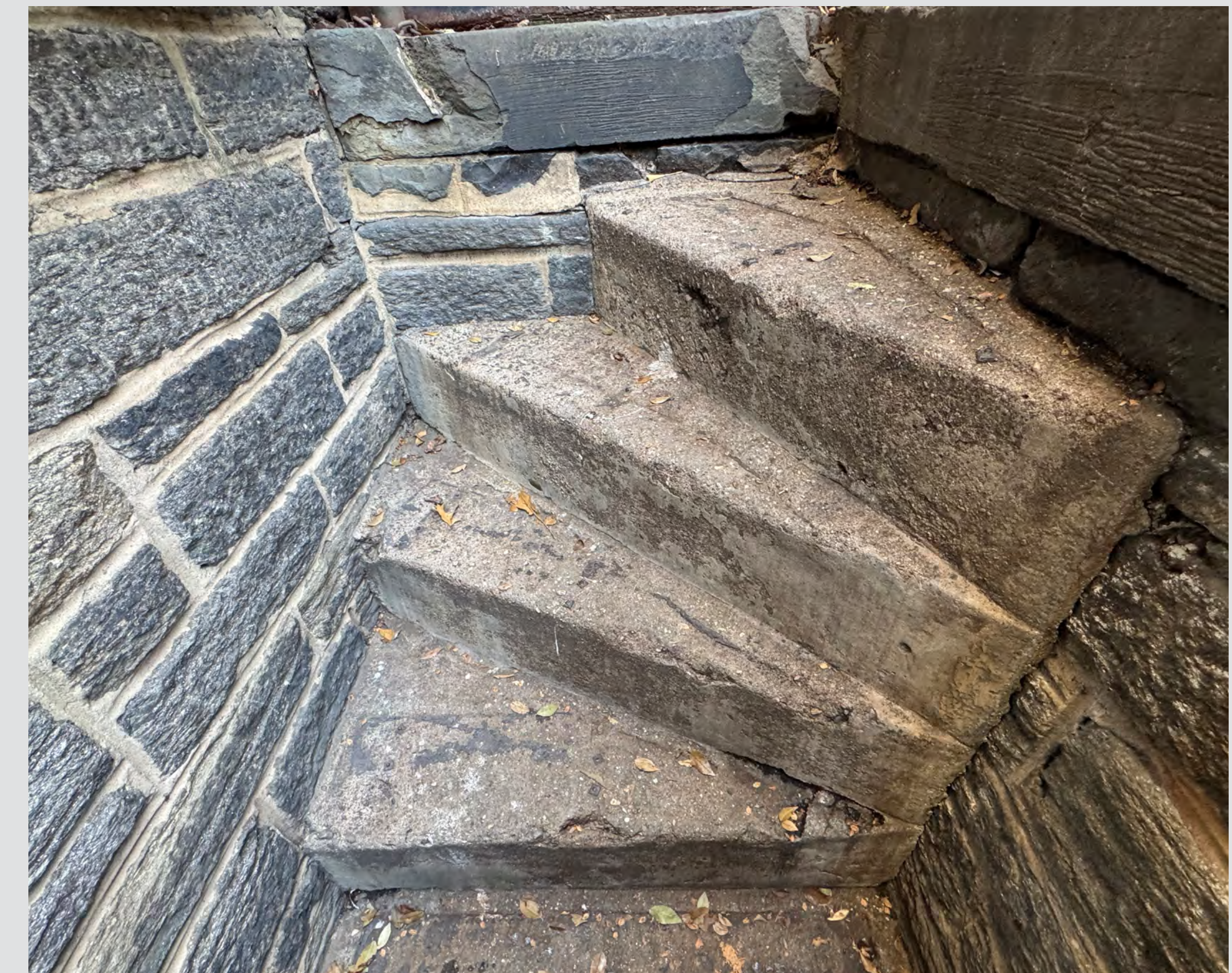
③ DETAIL OF CONCRETE STEPS TO THE BASEMENT. TOP FOUR STEPS NEED TO BE MODIFIED TO REACH LEVEL OF THE PROPOSED RAMP
